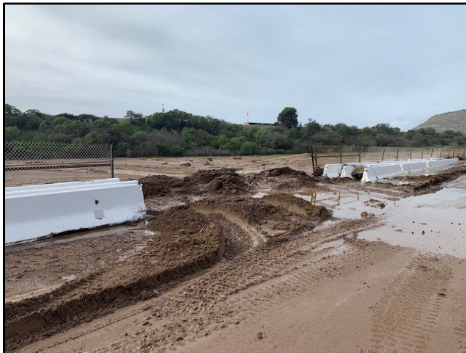
Figure 7-3. Onshore Facility Damage Following January 2023 Storm Event
