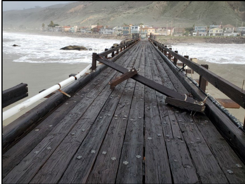
Figure 7-2. Rincon Causeway Storm Damage Following January 2023 Storm Event
