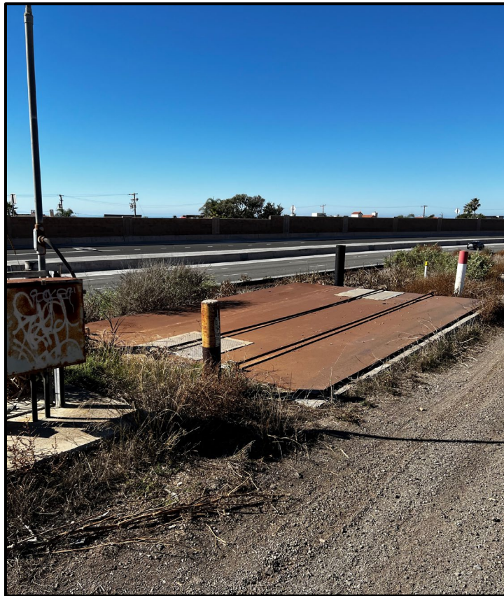
Figure 2-11. Onshore Pipeline Connections Vault Box Area North of U.S. Highway 101
