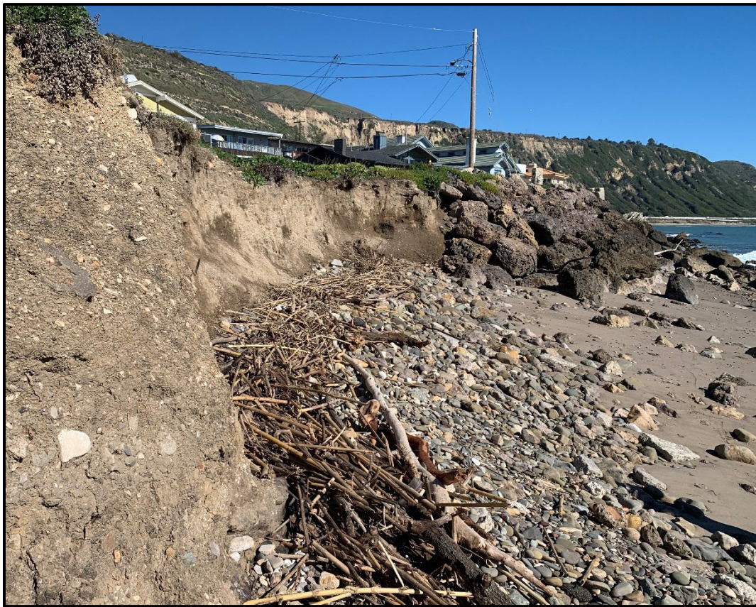
Figure 4.6-3. View of Upper Portion of SCC Parcel and Bluff Erosion (2024)
