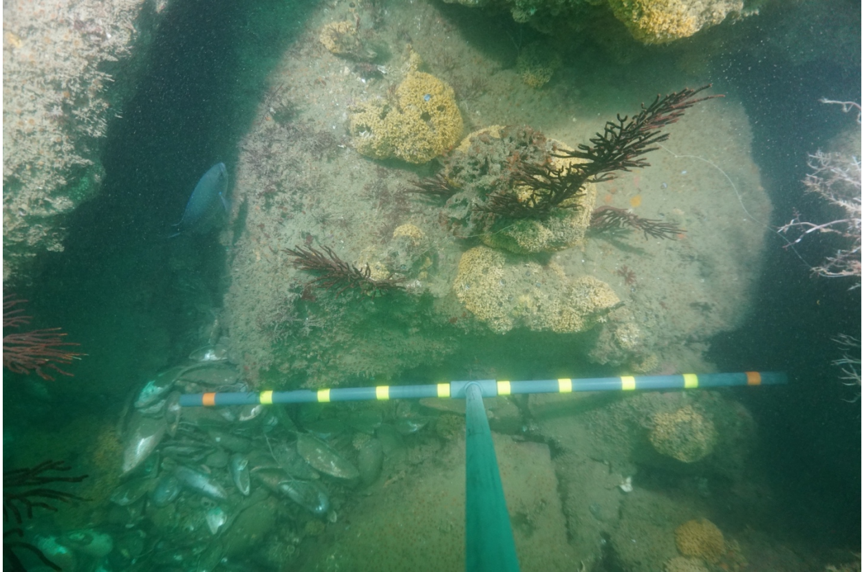
Figure 20. Base of the Armor Revetment on West Side of Rincon Island
