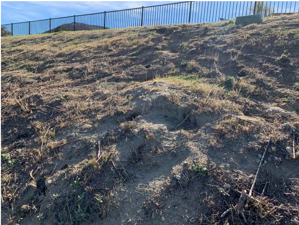
Photograph 4: Exposed clay contaminated soils with gravel on the southern slope of the basin.
