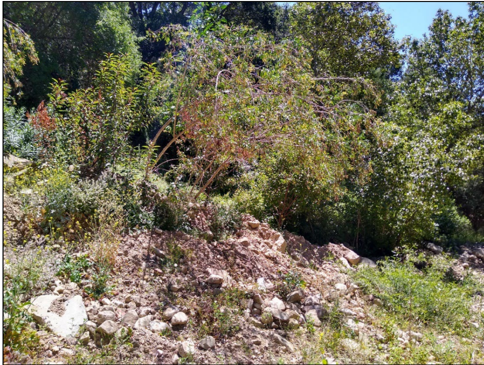
Photo 9. View of the vegetation present on the southeast side of the culvert facing northeast.
