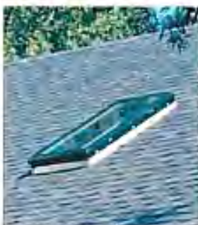
Use bar skylights; plastic will melt and allow embers into the home.
