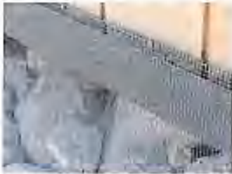
Cover openings with 1/8" metal screen to block fire brand and ember from collecting under the home or deck.
