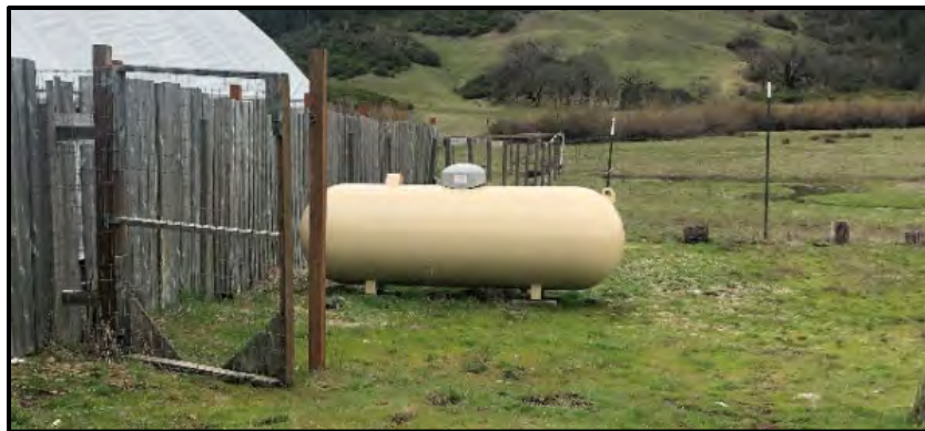
Figure 25- A Propane Tank Identified on the Property.
