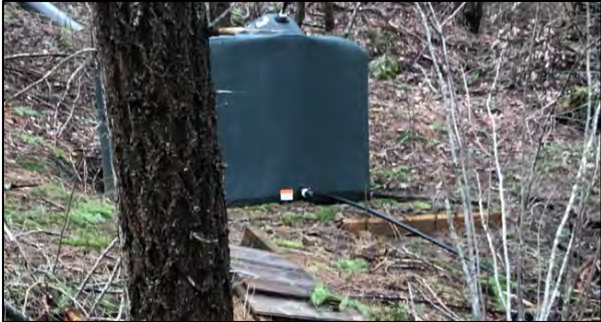
Figure 20- One of the Water Storage Tanks Identified Adjacent to the Access Road Leading to the Spring.
