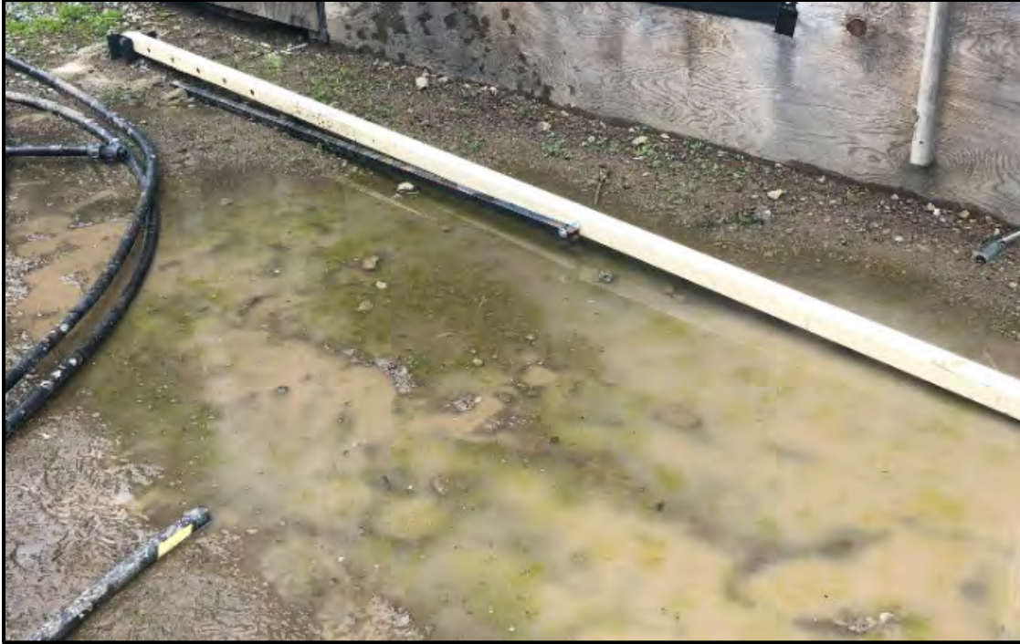
Figure 24- Standing Water on the Property with Evidence of Irrigation Runoff.
