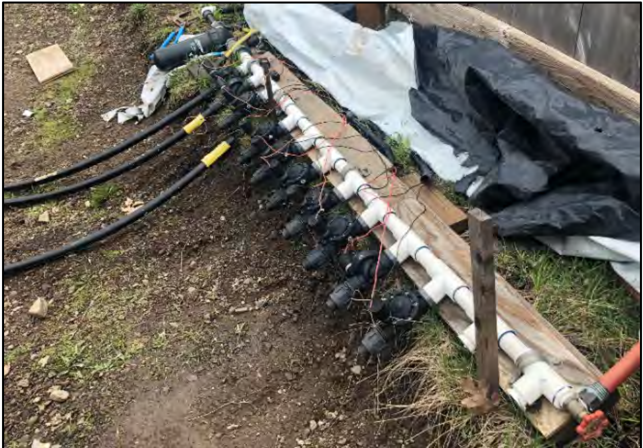
Figure 23- An Irrigation Manifold Identified on the Property.
