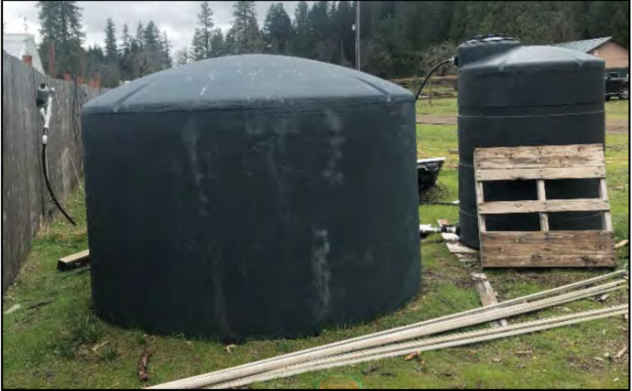
Figure 18- Water Storage Tanks Identified on the Property.
