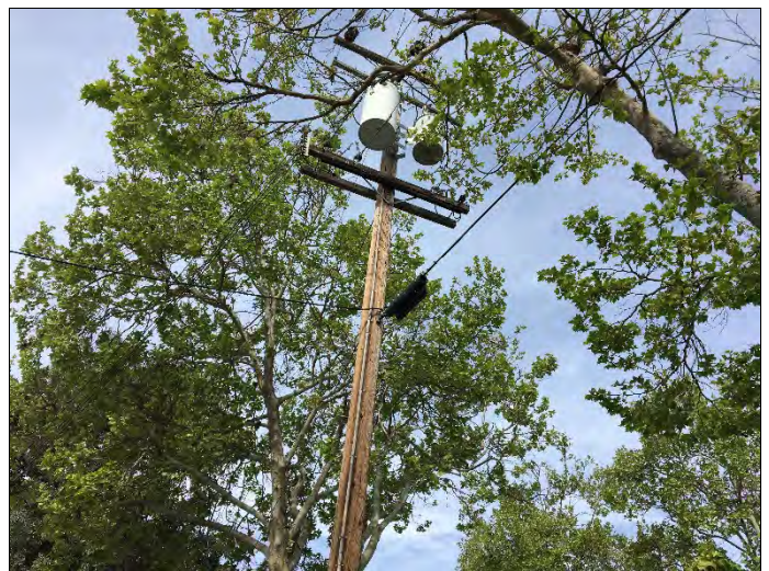
6. View of pole-mounted transformer.
