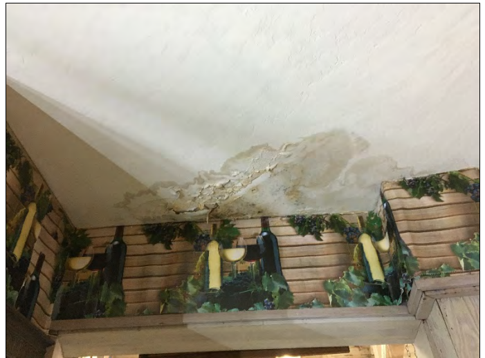
10. View of water intrusion.
