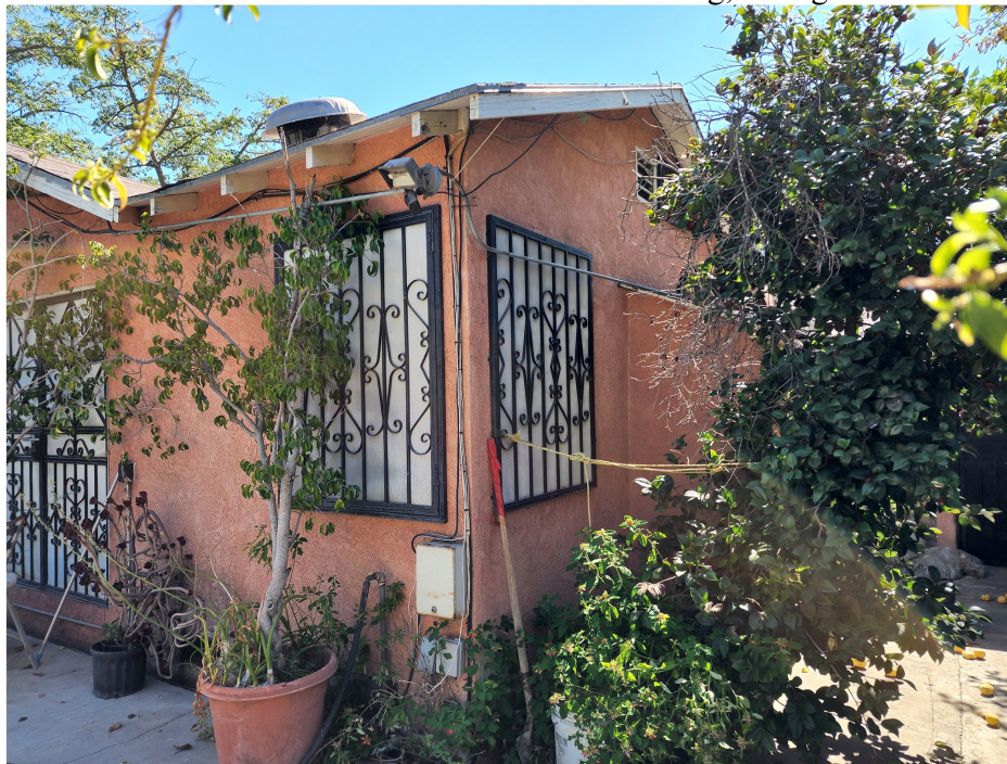
Plate 3.3-55: East (left) and north (right) façades of the 1985 to 1994 addition to the 16204 Santa Ana Avenue building, facing southwest.
