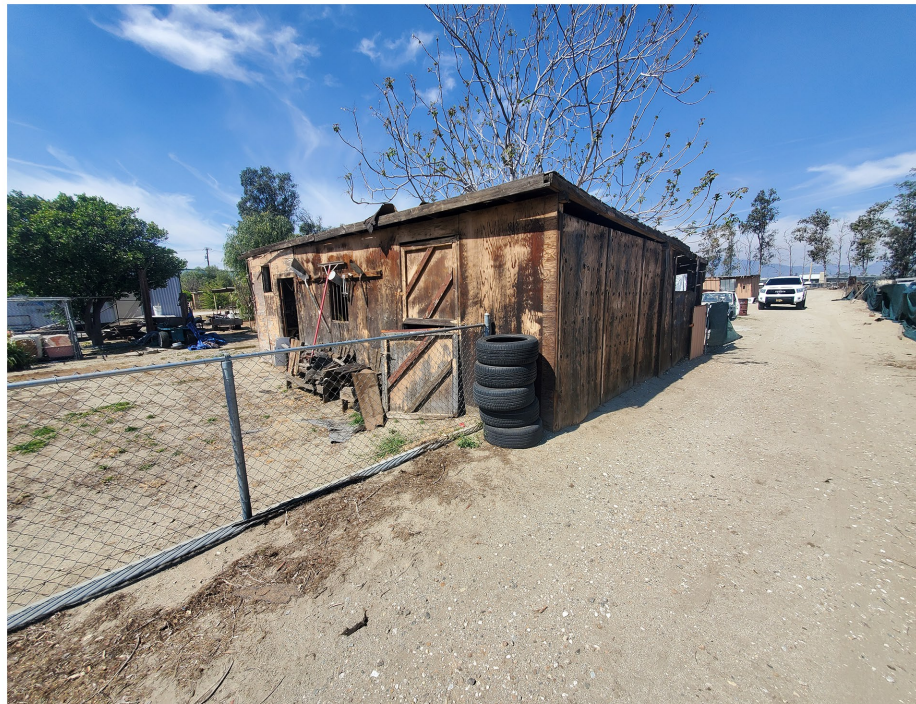
Plate 3.3–43: South (left) and east (right) façades of the wood-framed structure behind the 16156 Santa Ana Avenue building, facing northwest.
