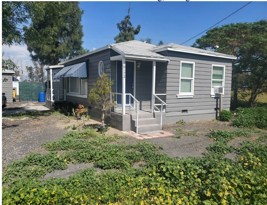
Plate 3.3–45: West (left) and south (right) façades of the 16172 Santa Ana Avenue building, facing northeast.
