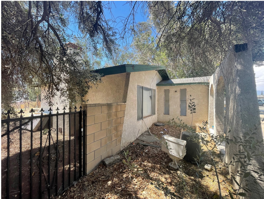
Plate 3.3-13: Southern portion of the east façade of the 10818 Oleander Avenue building, facing north.
