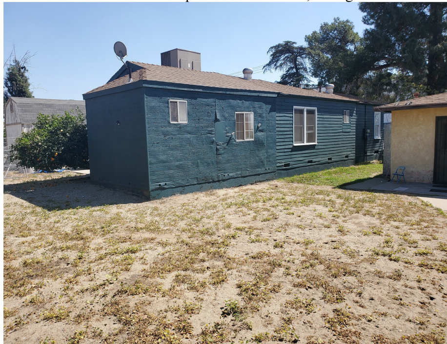
Plate 3.3–35: North (left) and west (right) façades of the 16140 Santa Ana Avenue prefabricated home, facing southeast .
