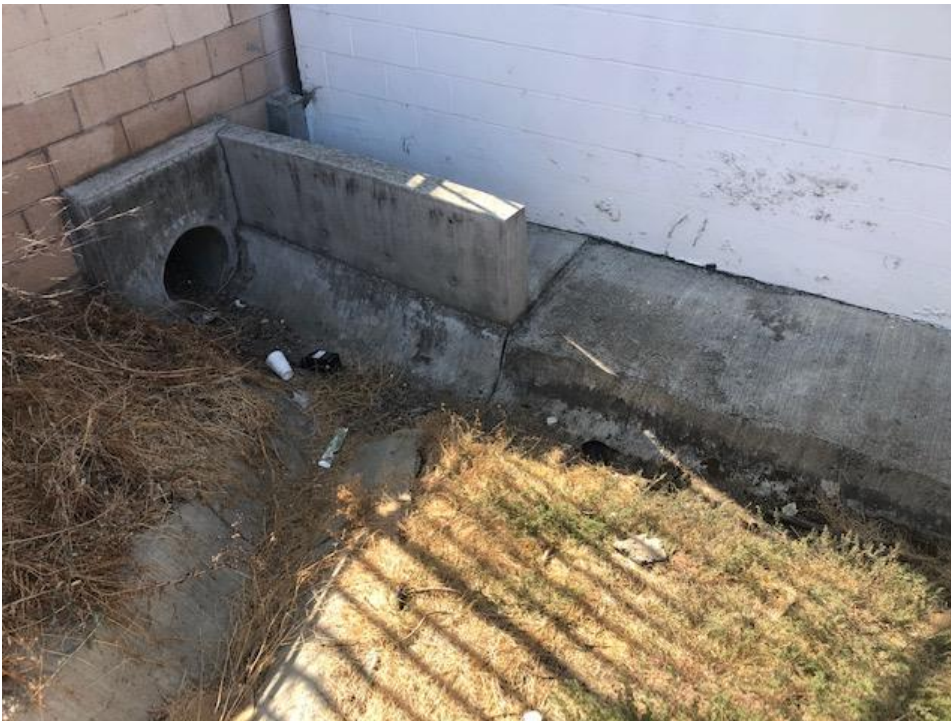
Photograph 4. Photo showing the culvert on the southeast corner of the site that directs stormwater off site.
