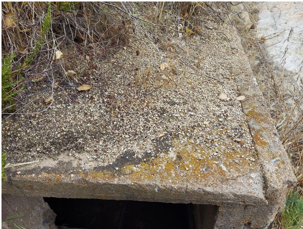
Concrete cover on top of cistern on downstream side. View to the east.
