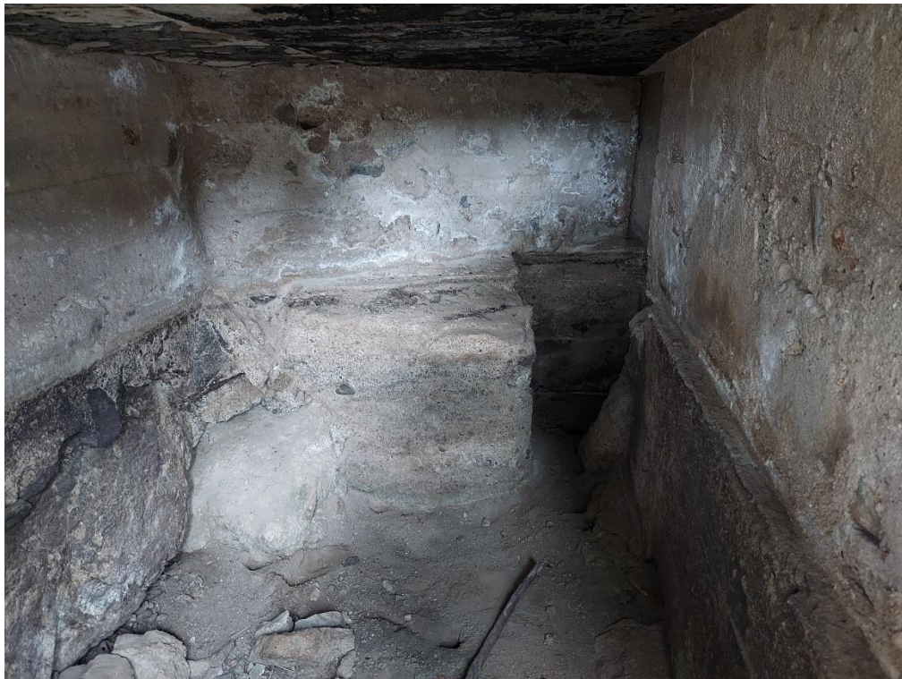
Inside walls of concrete cistern. Vertical pipe in far-right corner is not visible. View to the east.
