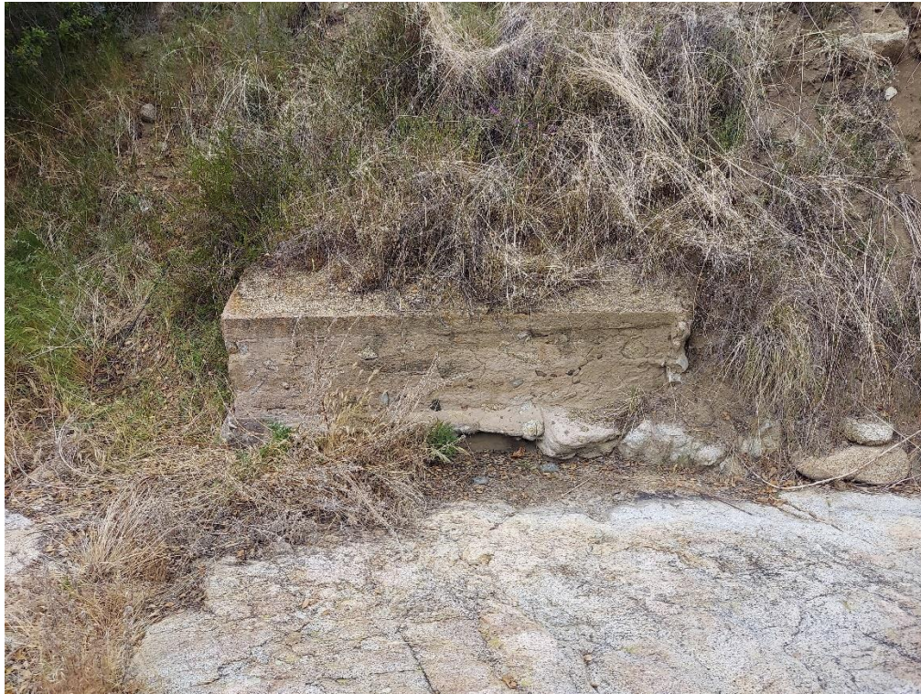
Concrete cistern near edge of intermittent creek and east of basin reservoir. View to the north
