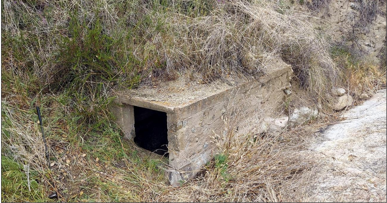
Figure 10. Concrete cistern at Site 3684-04H. (View to the northeast; photograph taken on April 13, 2021)
