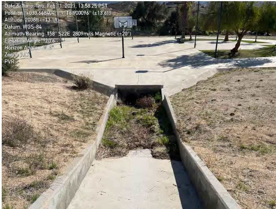
PHOTOGRAPH 9: A concrete channel leading down to the culverts of Feature A 2 under the sports complex.
