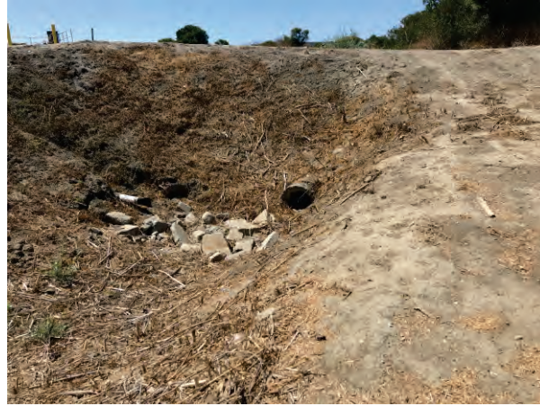
Photo 14. View of culvert #3 within the irrigation canal that connects to the Salinas River, facing southwest. August 11, 2022
