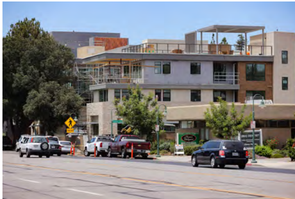
The luxury apartment complex rises above E. Thousand Oaks Boulevard across from Tarantula Hill Brewing Company. Residents are expected to begin moving in sometime in October. Two restaurants, Go Fish Sushi and JOi Cafe, have already signed on to fill the commercial spaces on the bottom floor facing. MICHAEL COONS/Acorn Newspapers
