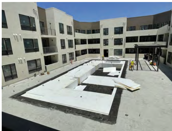
At the center of the future complex, an “upscale pool,” the developers said. The project also includes a rooftop terrace with firepit and lounge seating, a robust fitness center and various covered seating areas on the first and second floor. KYLE JORREY/Acorn Newspapers
