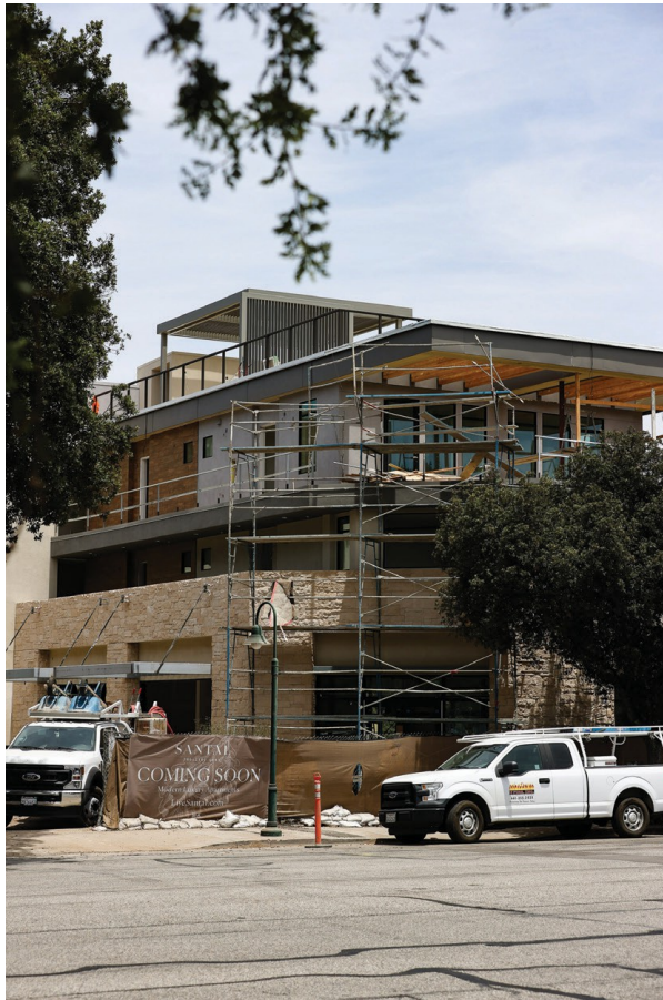
TOP OF THE CITY—Construction is nearing completion at 299 E. Thousand Oaks Blvd. The mixed-use development features 142 units, 11 of which have been designated as “affordable” and will be leased for significantly less than the 131 market-rate apartments. MICHAEL COONS Acorn Newspapers
