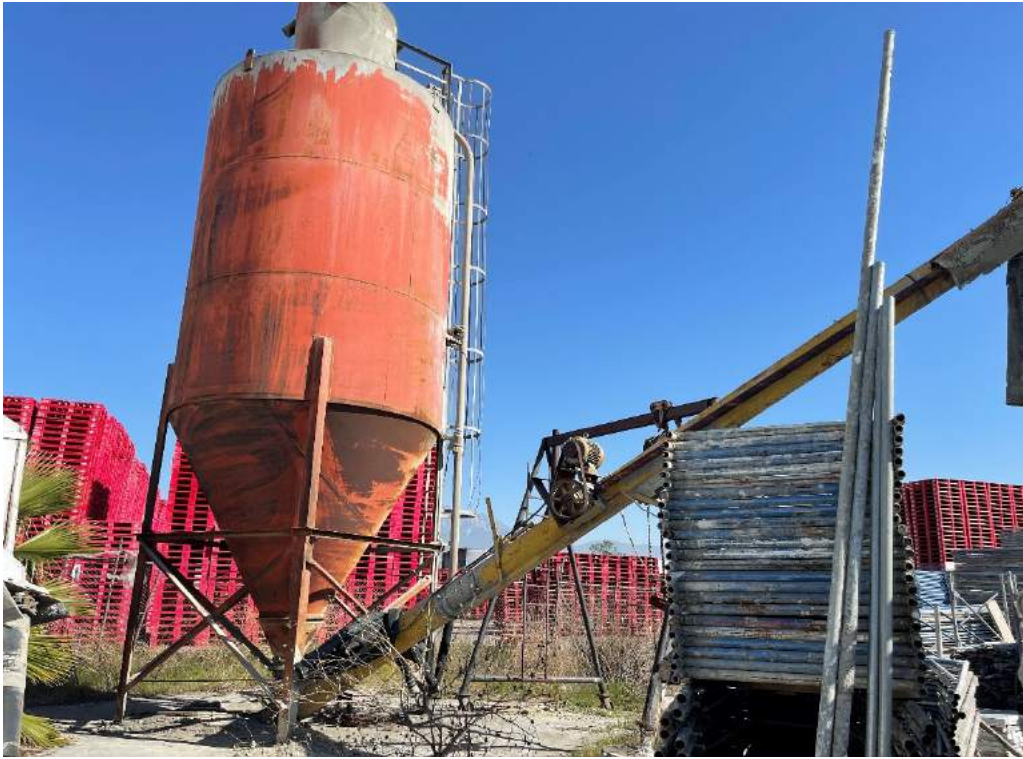
Photo 11: Abandoned AST on northwest corner of the site.
