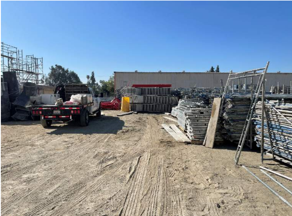
Photo 7: Exterior storage on unpaved surface on central portion of the site.
