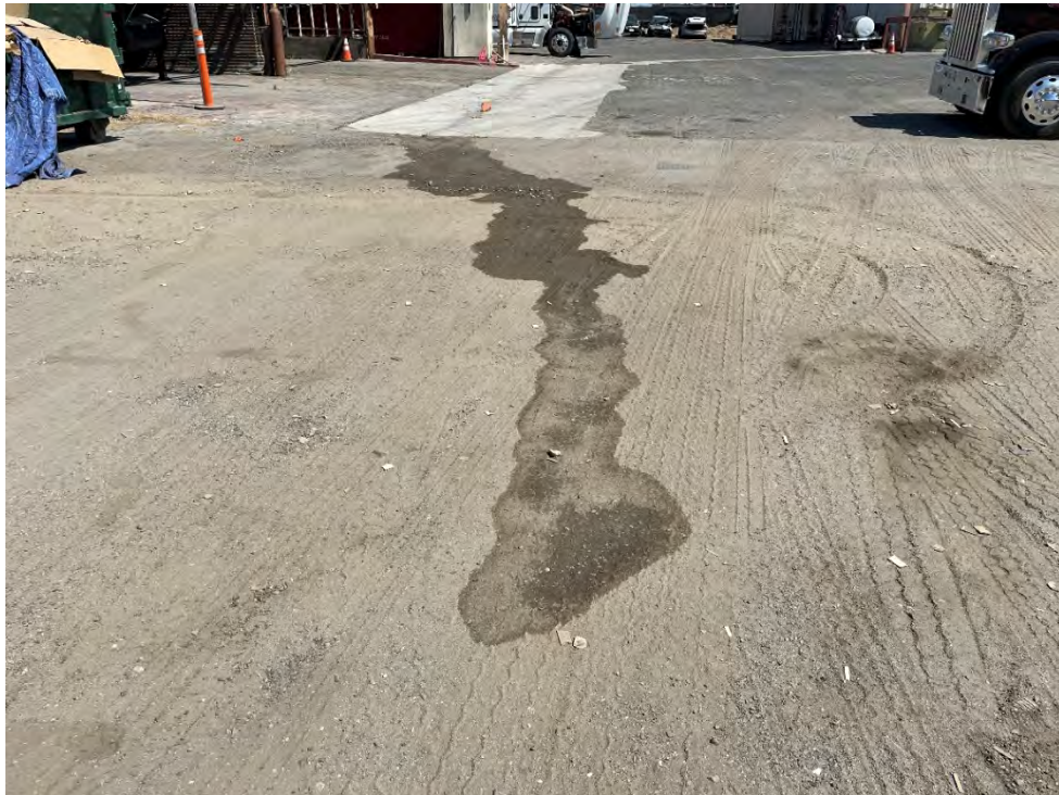
Photo 4: View of a surficial stain located on an unpaved surface in the western portion of the site.
