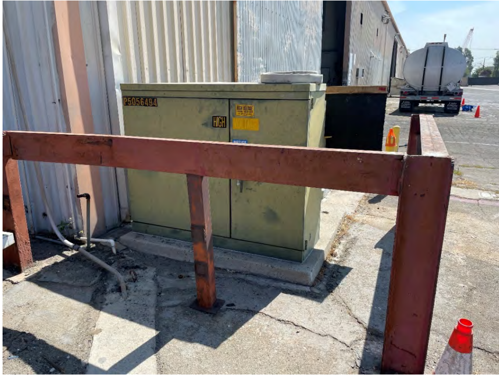
Photo 11: View of the pad-mounted transformer located to the southwest of the warehouse.
