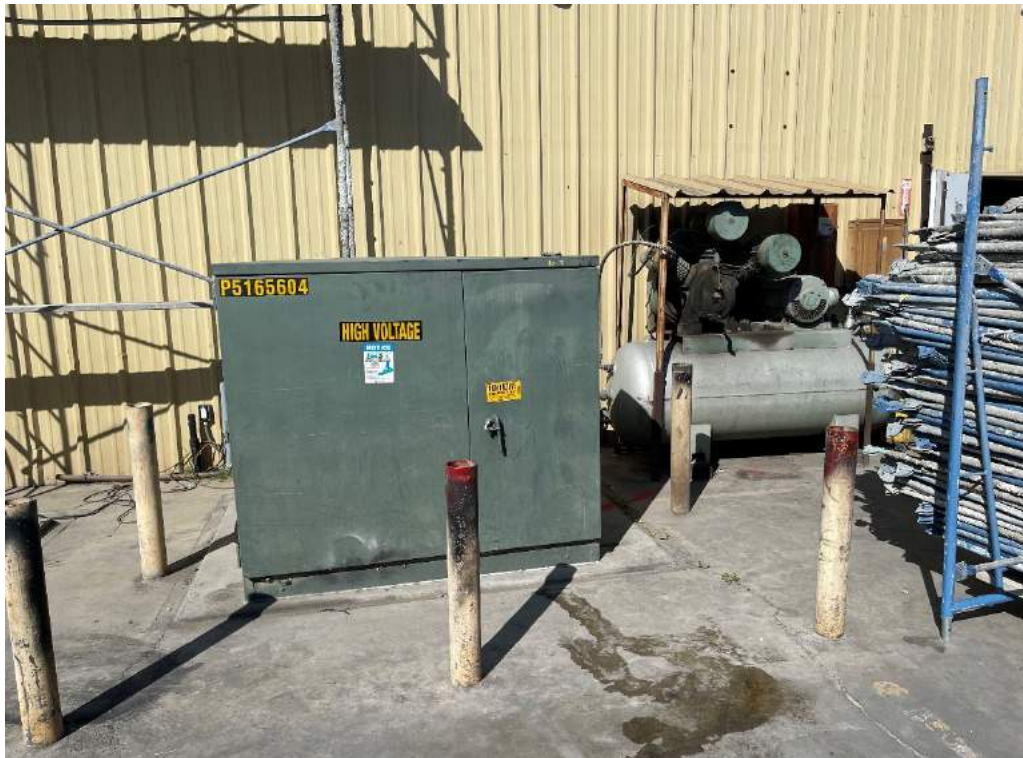
Photo 9: Pad-mounted transformer and air compressor outside eastern wall of warehouse building.
