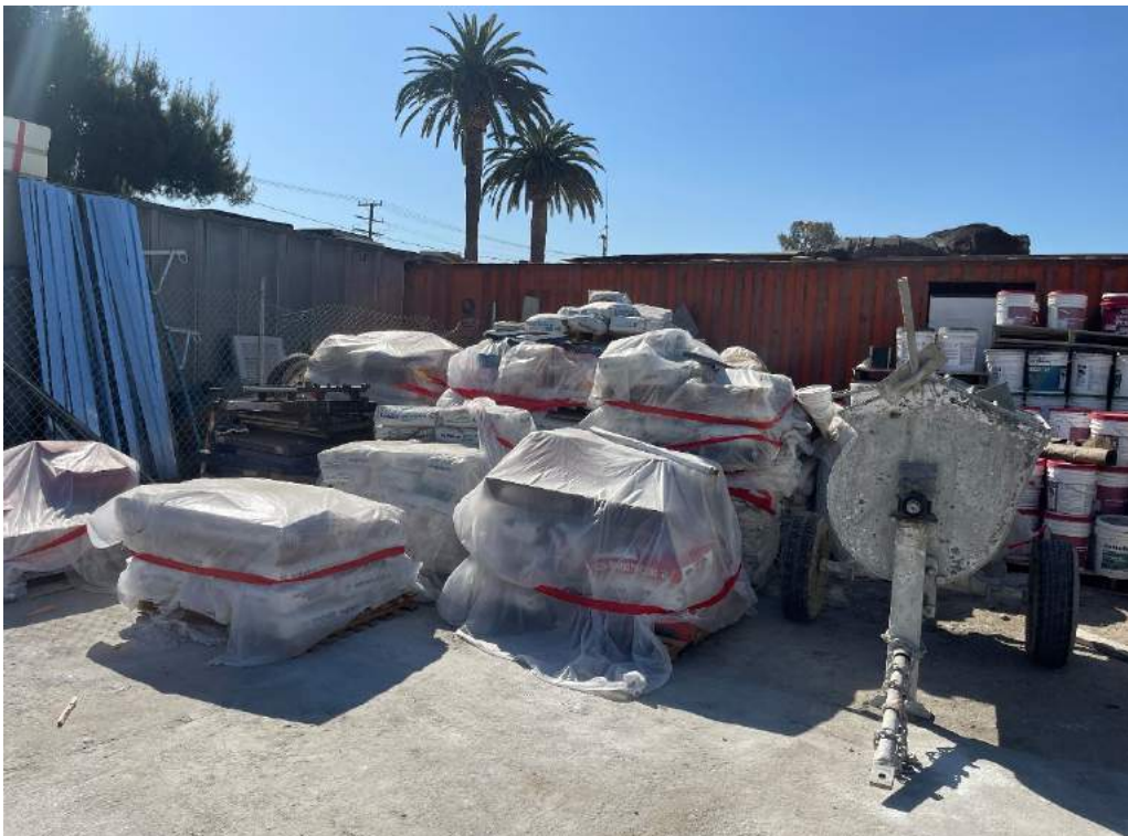
Photo 6: Outdoor storage of plaster mix, acrylic primer, and acrylic finish and plaster mixing machine.
