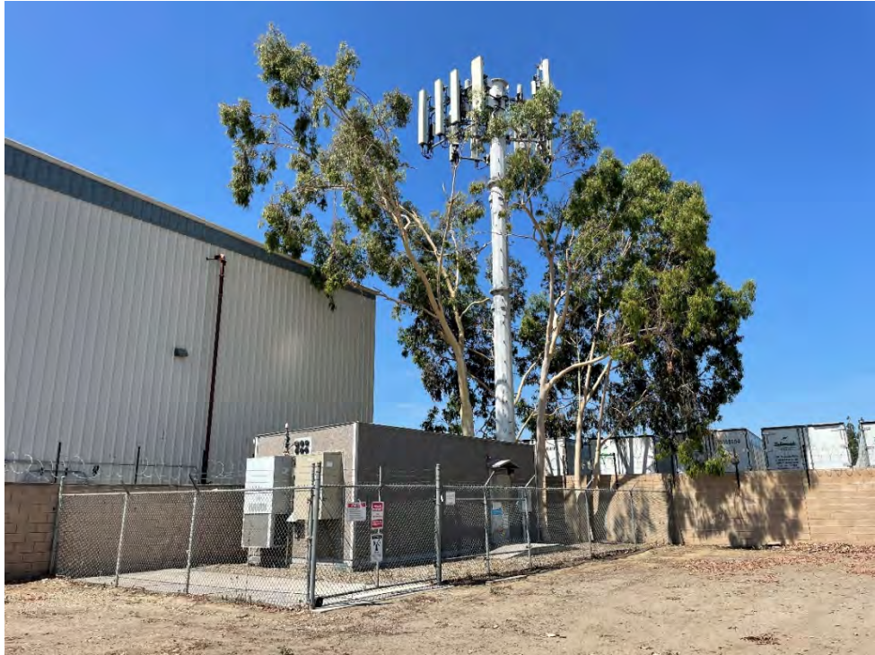
Photo 3: View of the AT&T cell tower on the southwest corner of the site, from the north.
