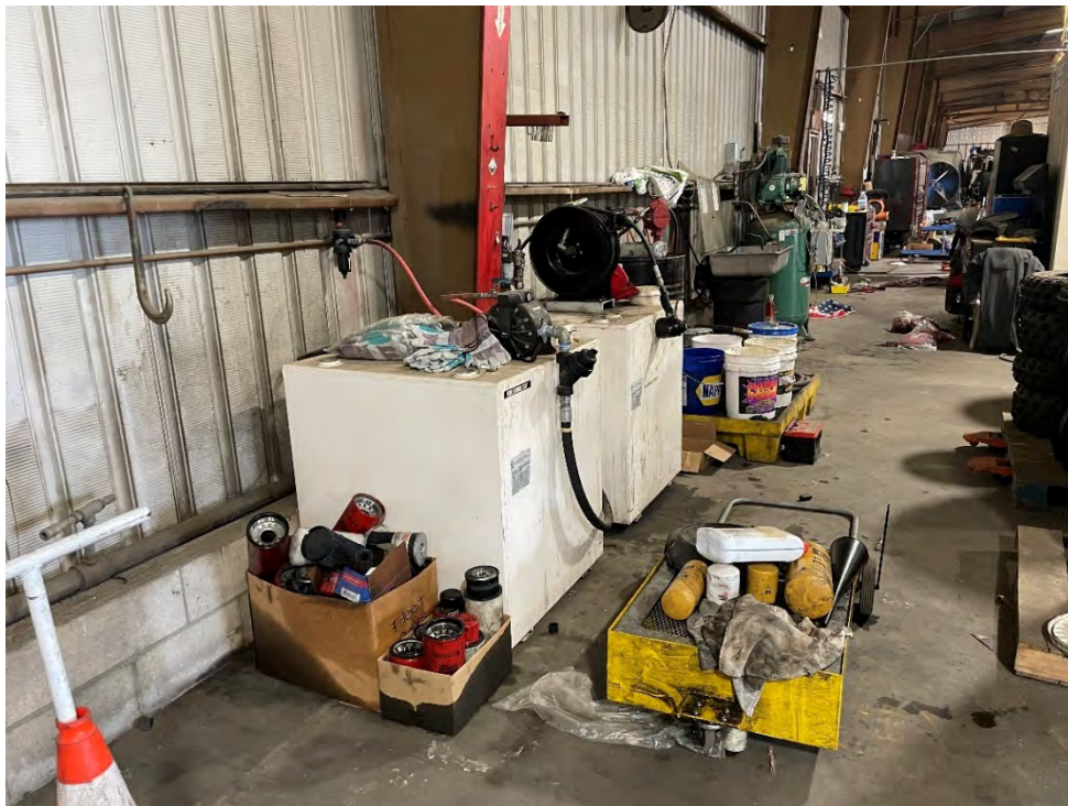
Photo 8: View of the oil ASTs located in the northern portion of the warehouse.
