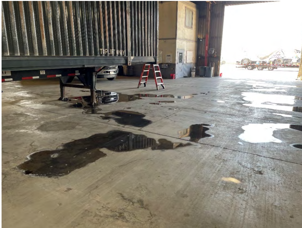
Photo 7: View of the pools of water located in the vehicle washing area in the western portion of the warehouse.
