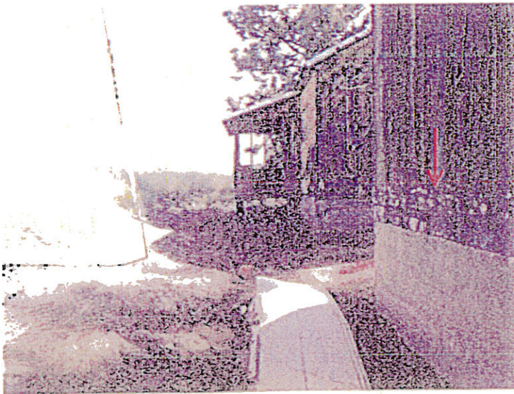
Photograph 2. View looking east of the existing building in the eastern portion of the study area, showing water marks, identified by the red arrow, on the buildings and the 4–6 feet of fill placed around the buildings.
