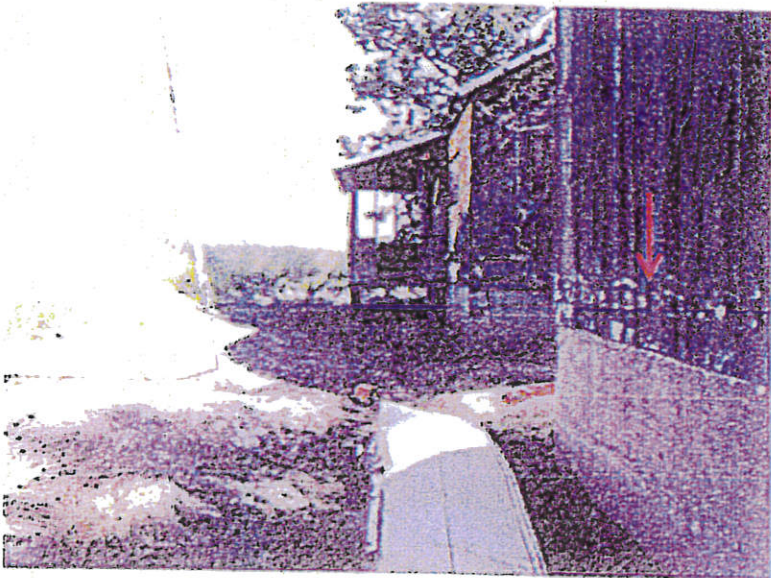
Photograph 2. View looking east of the existing building in the eastern portion of the study area, showing water marks, identified by the red arrow, on the buildings and the 4–6 feet of fill placed around the buildings.
