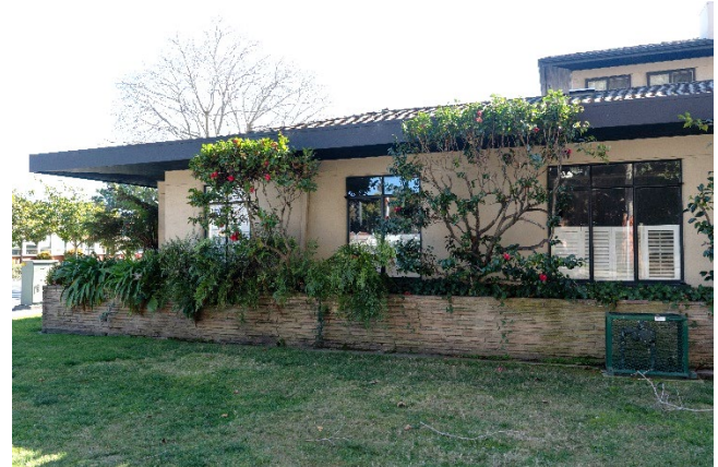
Figure 4: Typical window arrangement, shown here at north end of west façade. Looking northeast.
