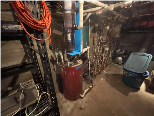
Photo 9: Amalgam separator in basement of 680 University Avenue.
