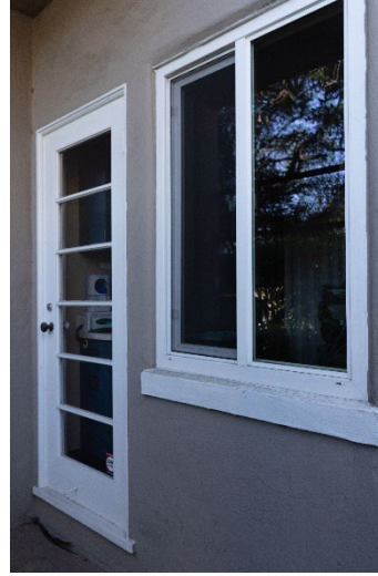
Figure 7: Door at west end of east section of rear façade. Looking southeast.
