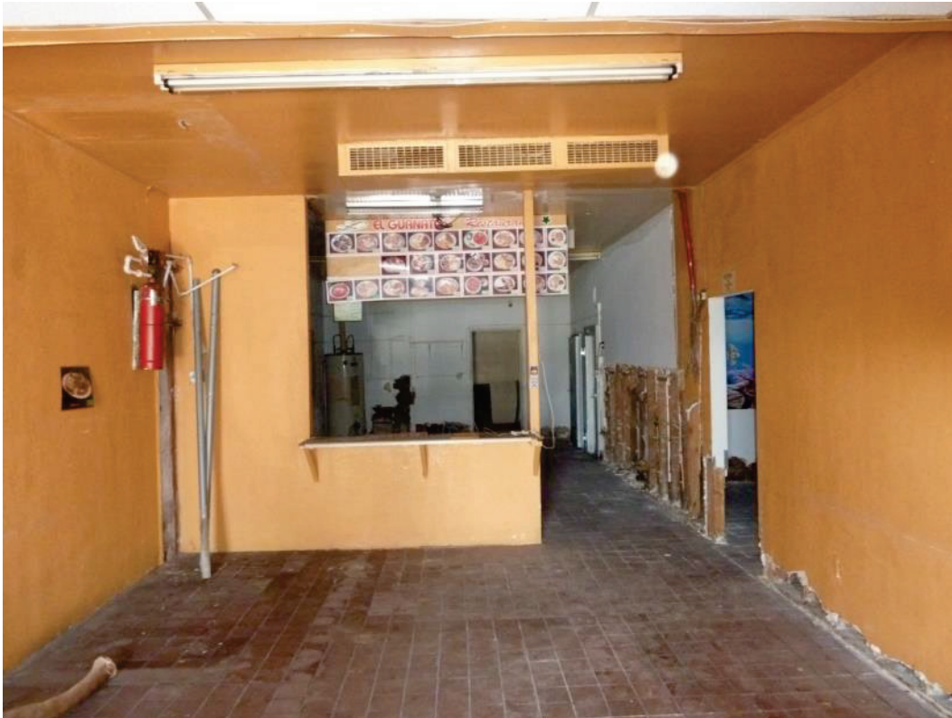
F-34. Interior of former restaurant 11540 Alondra with opening in wall at right to 11538 Alondra (7/10/2014).
