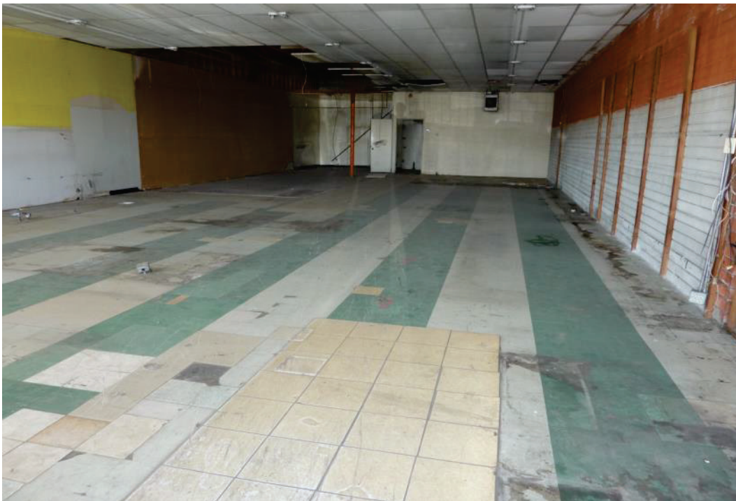
F-14. Interior of former convenience store at 11524 Alondra with portion of ceiling missing (7/10/2014).
