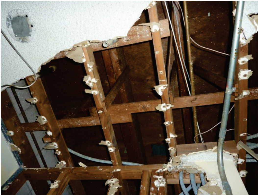
F-35. Damaged ceiling with textured finish exposing underside of uninsulated roof in former restaurant at 11540 Alondra (7/10/2014).
