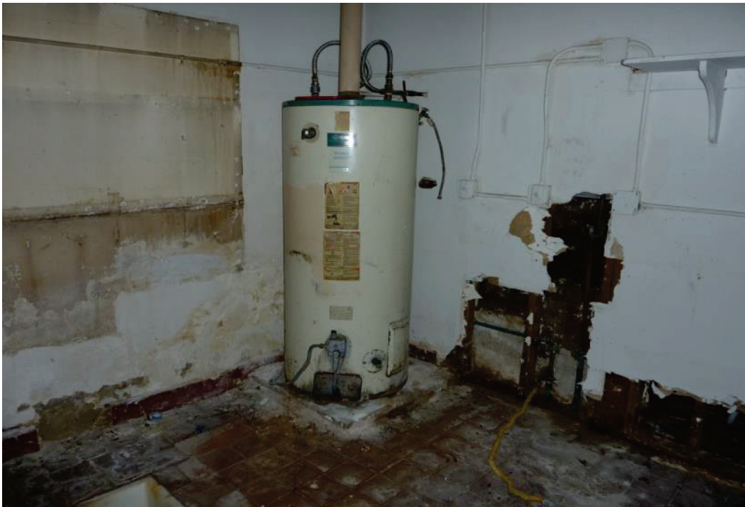
F-36. Water heater inside former restaurant at 11540 Alondra with ceramic floor tile in foreground (7/10/2014).
