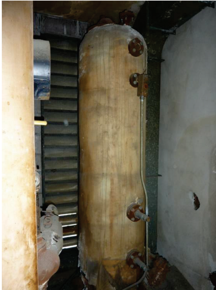
F-31. Hot water tank with suspected asbestos insulation on mezzanine inside former Thrifty drug store at 11536 Alondra (7/10/2014).
