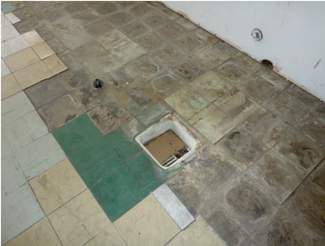
F-15. Floor drain inside former convenience store at 11524 Alondra (7/10/2014).
