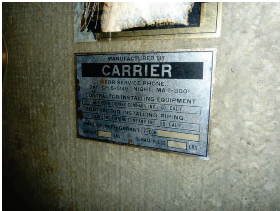
F-32. Air conditioning unit containing Freon refrigerant on mezzanine inside former Thrifty drug store at 11536 Alondra (7/10/2014).
