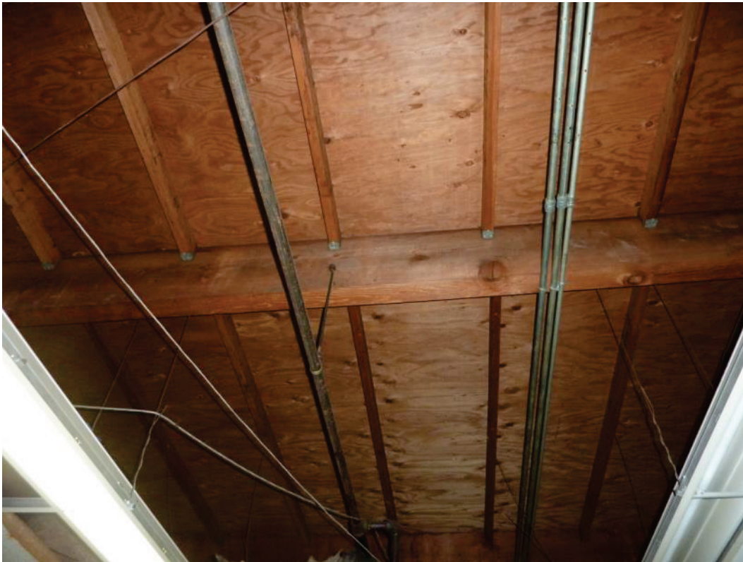
F-39. Underside of uninsulated roof on mezzanine inside Norwalk Indoor Swap Meet at 11600 Alondra (7/10/2014).
