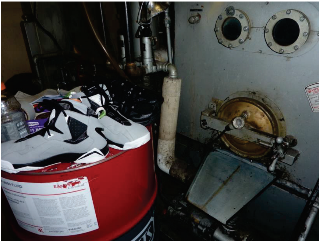
F-18. Boiler with dry cleaning machine in background and 55-gallon drum of ExxonMobil DF-2000 in foreground at Deluxe Cleaners at 11526 Alondra (7/10/2014).
