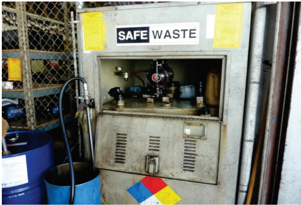
F-7. Waste oil storage tank at Rusty's Automotive, 11522 Alondra (7/10/2014).
