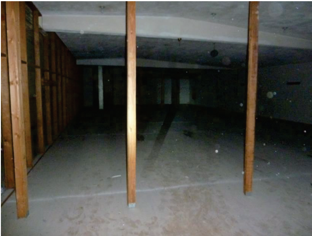
F-30. Stock room on mezzanine inside former Thrifty drug store at 11536 Alondra (7/10/2014).
