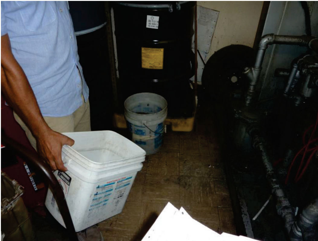
F-19. Dry cleaning machine and 55-gallon drum of spent solvent at Deluxe Cleaners at 11526 Alondra (7/10/2014).
