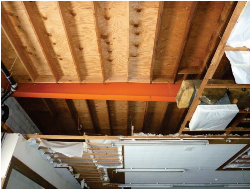
F-29. Underside of uninsulated roof inside former Thrifty drug store at 11536 Alondra (7/10/2014).
