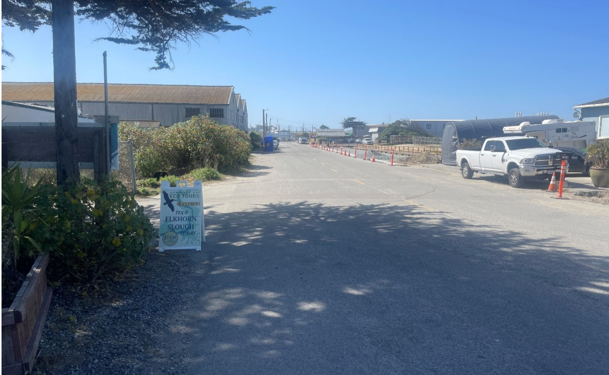
Photograph 7. Location of Pipe Repair P-1 within developed land cover, facing south April 8, 2022.
