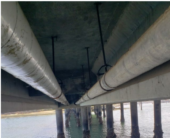
Photograph 5. Lift Station No. 2 Force Main under Elkhorn Slough Bridge
