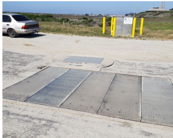
Photograph 4. Lift Station No. 4
