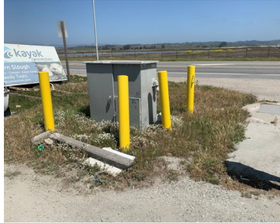
Photograph 2. Lift Station No. 2
