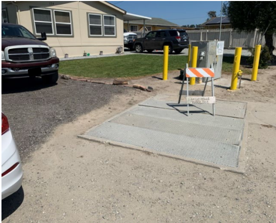
Photograph 1. Lift Station No. 1
