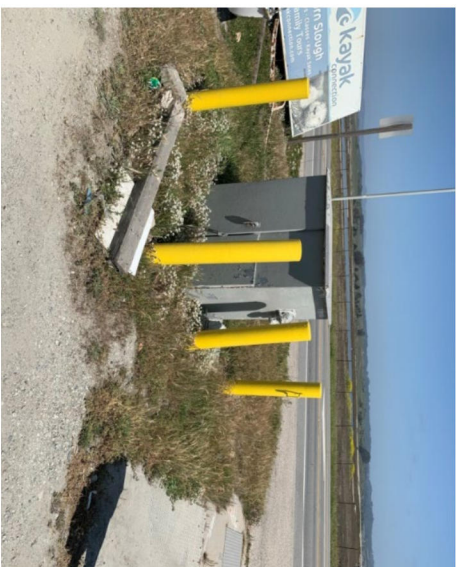
Photograph 2. Lift Station No. 2
