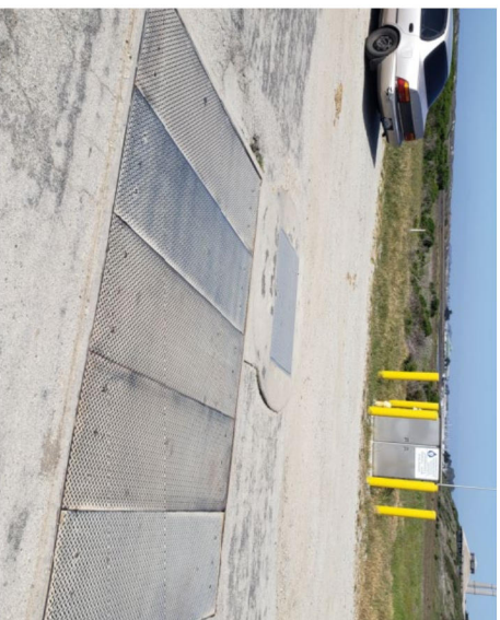
Photograph 4. Lift Station No. 4
