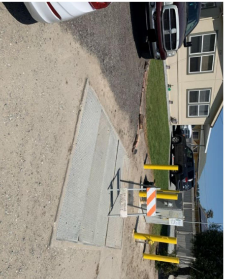
Photograph 1. Lift Station No. 1
