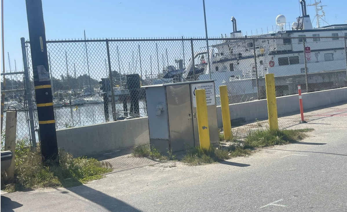
Photograph 5. Lift Station No. 3 within developed land cover, facing west. April 8, 2022.
