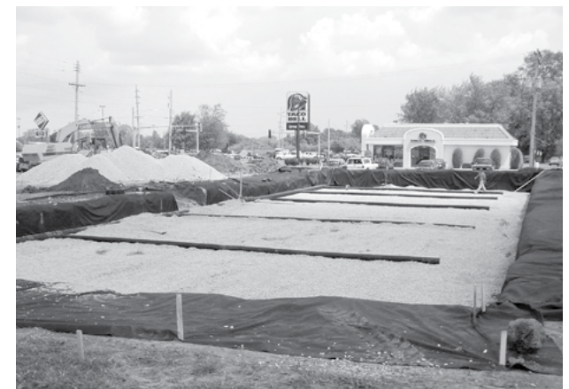
Place clean, crushed, angular stone foundation 9" (230 mm) min. Install underdrains if required. Compact to achieve a flat surface.
