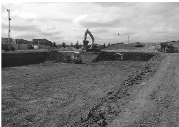
Excavate bed and prepare subgrade per engineer's plans. Plans and specifications should include Best Management Practices (BMPs) to deter contamination of open pits during construction.
