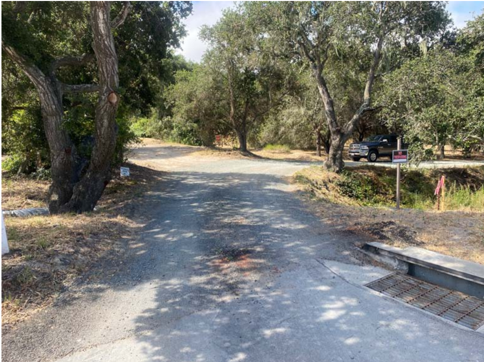
Photo 6. Southerly view of the northeastern corner of the study area taken from the end of Craig Way. A culvert is present under the access road and the storm drain inlet to the right directs road runoff into the swale. The access road to the site is on the right at the location of the truck. Road improvements may result in the removal of one of the oak trees at this location.
