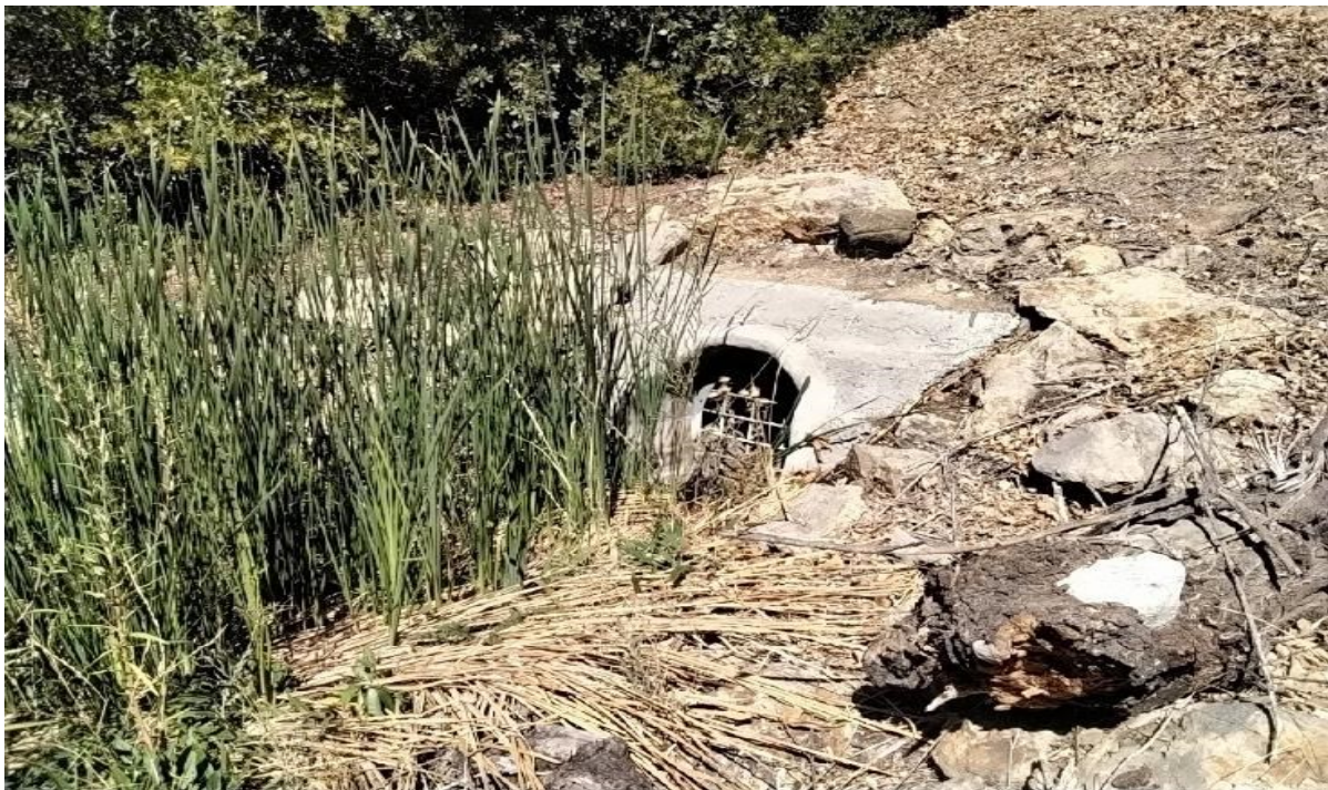
Photograph 31. View of Culvert Outlet 4 along the southwestern border of the Study Area, facing northwest (August 30, 2022).
