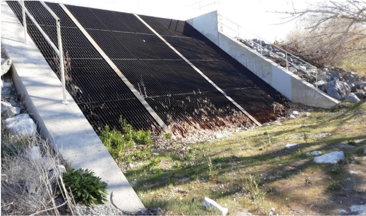
Photograph 9. Photo Point 9. View of the existing concrete outfall structure to the southeast and outside of the Study Area, facing northeast (February 23, 2022).
