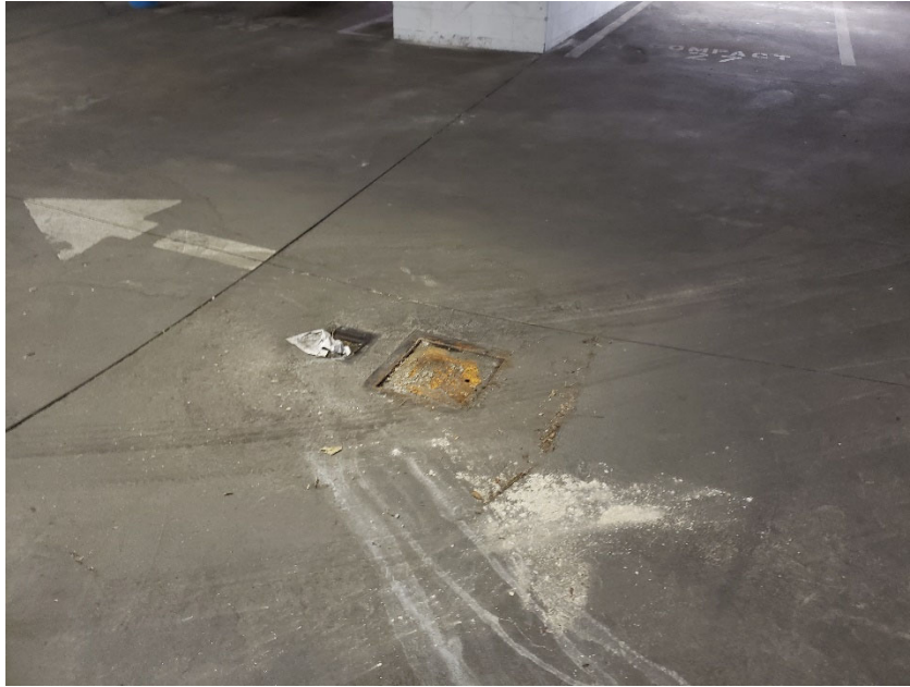
9. Sump at below-grade parking level at 6767 Sunset Boulevard
