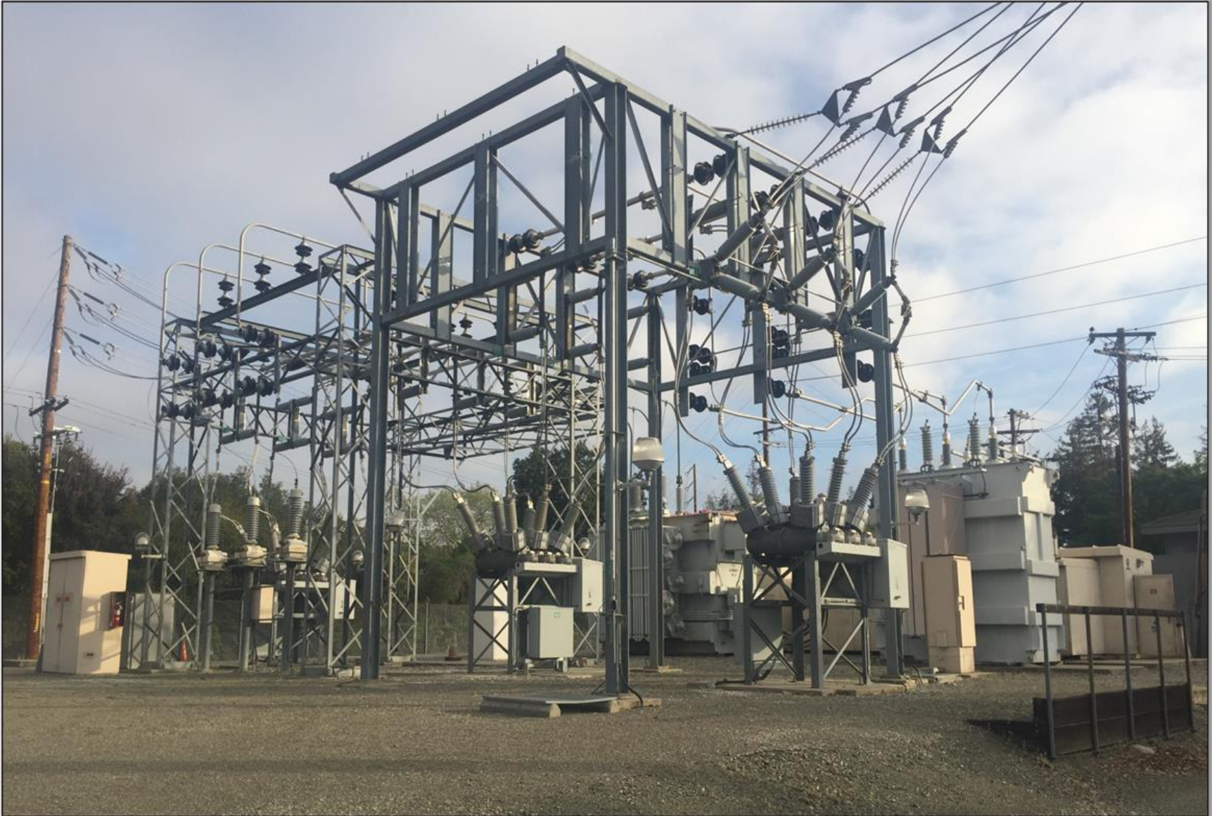
Figure 4.2 Existing Homestead Substation Looking Northeast
