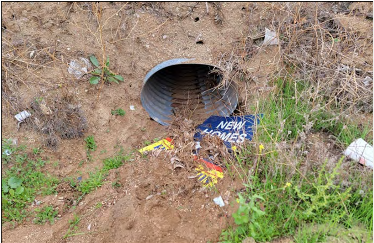
Photograph 15: View of western upstream 30-inch EF1 culvert on western side of Moreno Beach Drive, facing downstream and east. Culvert is proposed for complete removal, and an 18-inch storm drain to installed immediately north of this location.
