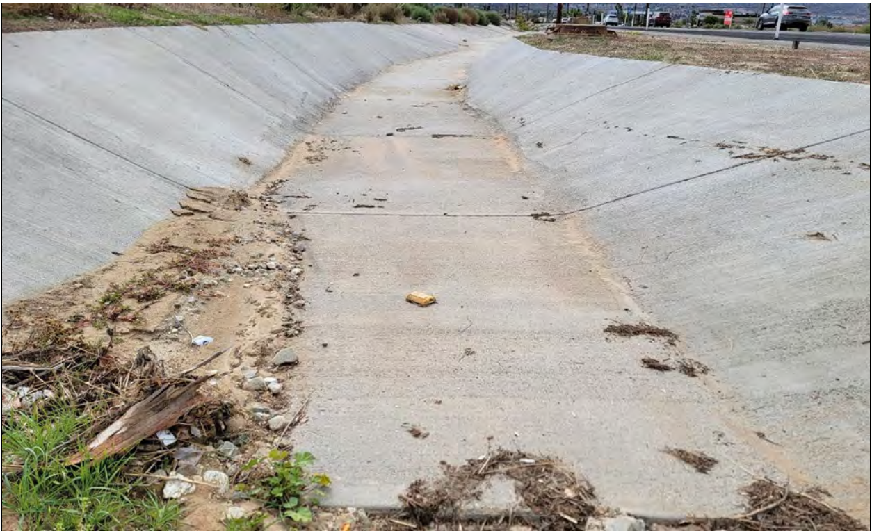
Photograph 17: View downstream and south of Drainage 4 south of Bay Avenue where the channel becomes a 5-foot wide concrete lined channel.
