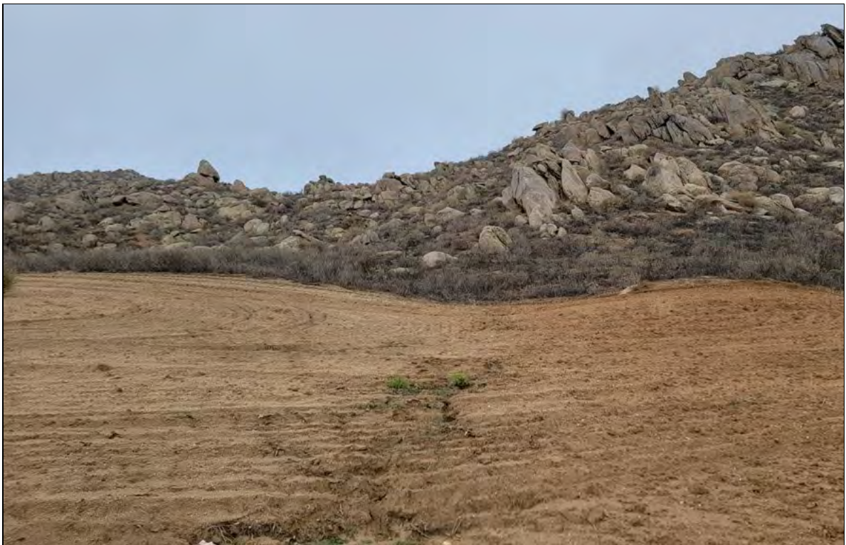
Photograph 14: View of erosional feature EF3 facing upstream and northwest from its intersection with Moreno Beach Drive.
