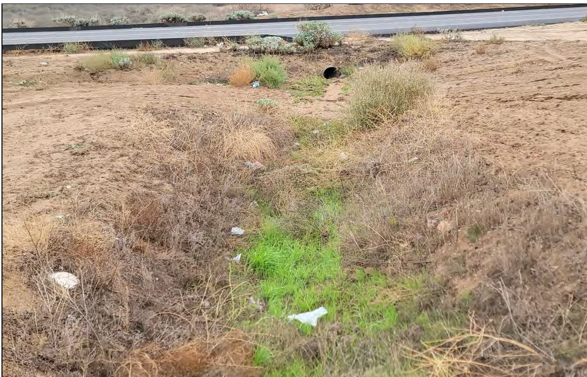
Photograph 10: View of erosional feature EF1, facing downstream and southeast towards its intersection with a metal culvert beneath Moreno Beach Drive.
