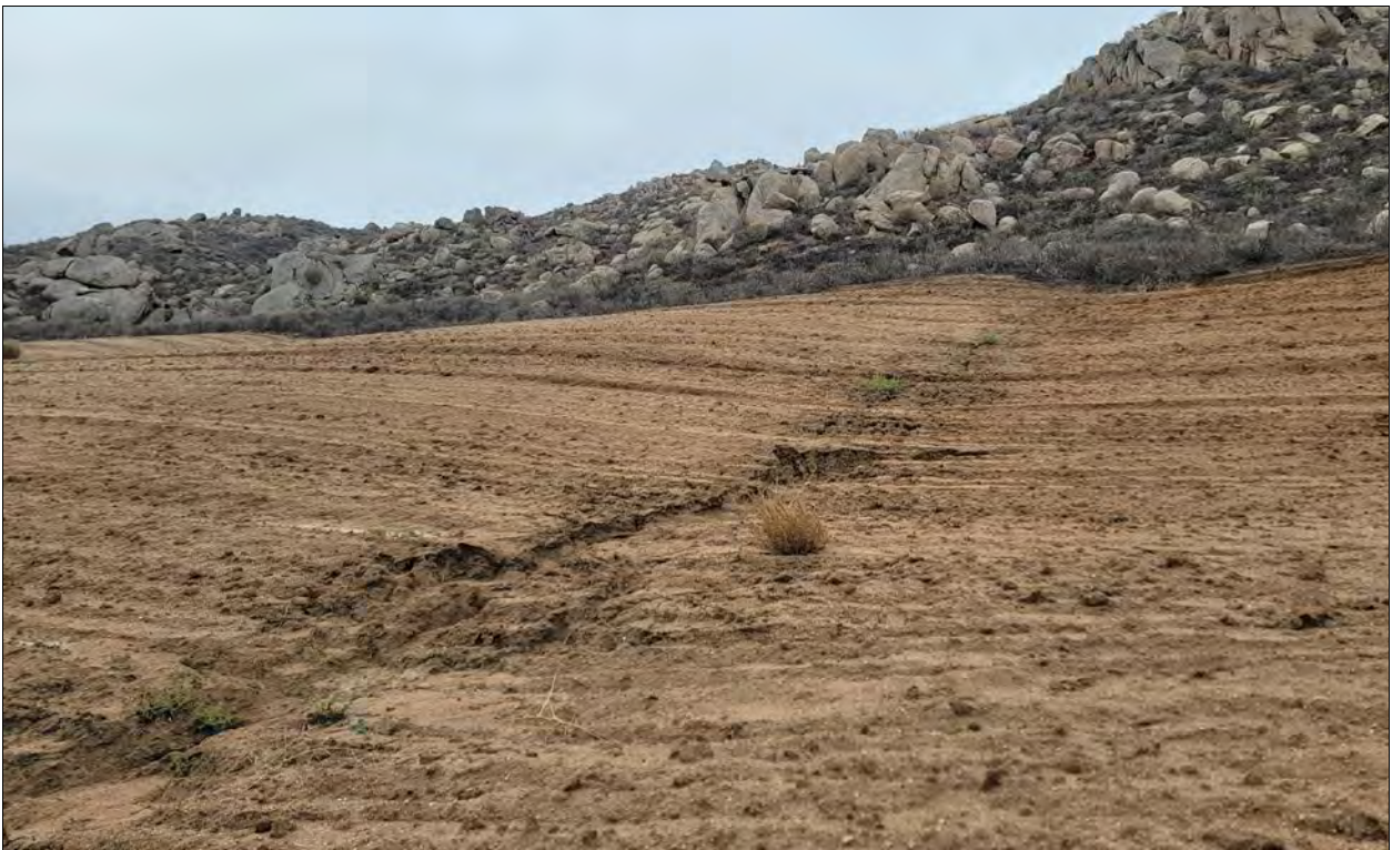
Photograph 6: View of Drainage 3 facing upstream and northwest from the northern boundary of the grading limits.
