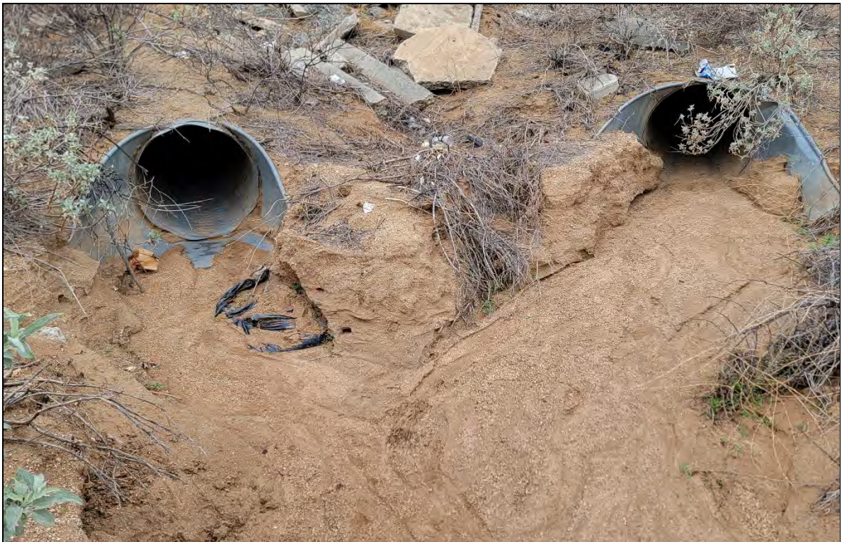
Photograph 20: View upstream towards two 30" culverts for EF2 (left) and EF3 (right), facing west, and their confluence just east of Moreno Beach Drive. Channel continues as a single ephemeral channel downstream conveying flows to the east.
