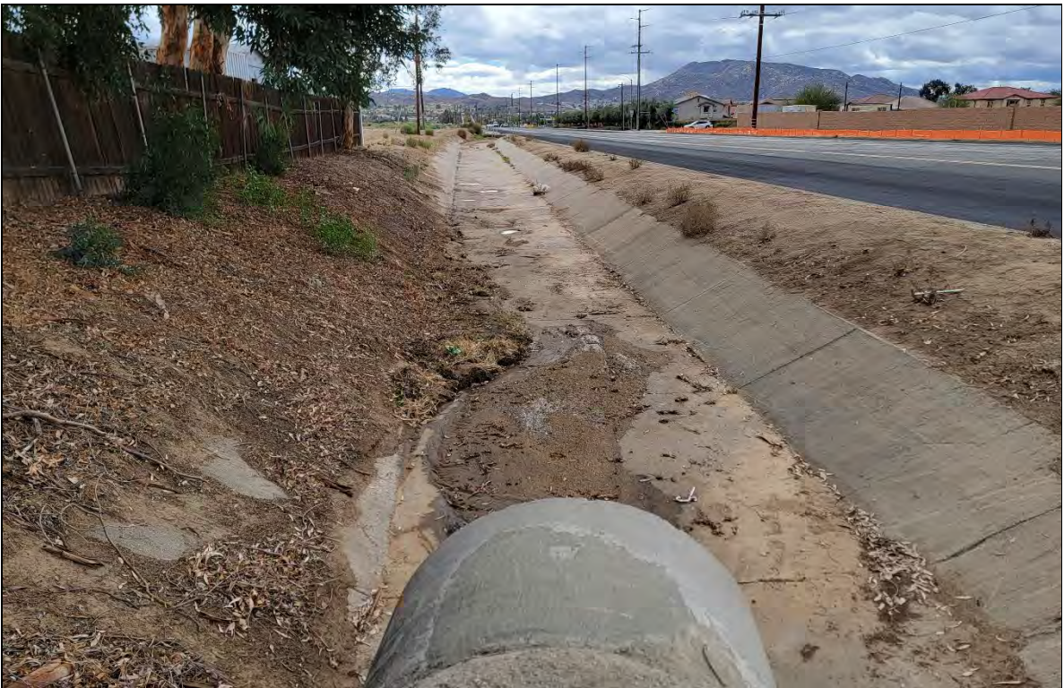
Photograph 22: View downstream from concrete culvert into 5-foot-wide concrete lined channel, facing south along Moreno Beach Drive.
