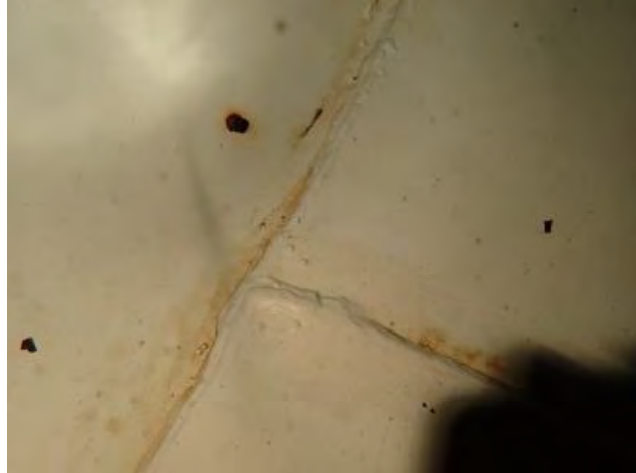
Figure 10: Floor plates with isolated corrosion spotting
