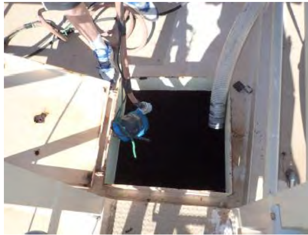
Figure 15: Roof hatch in moderate condition with areas of moderate corrosion
