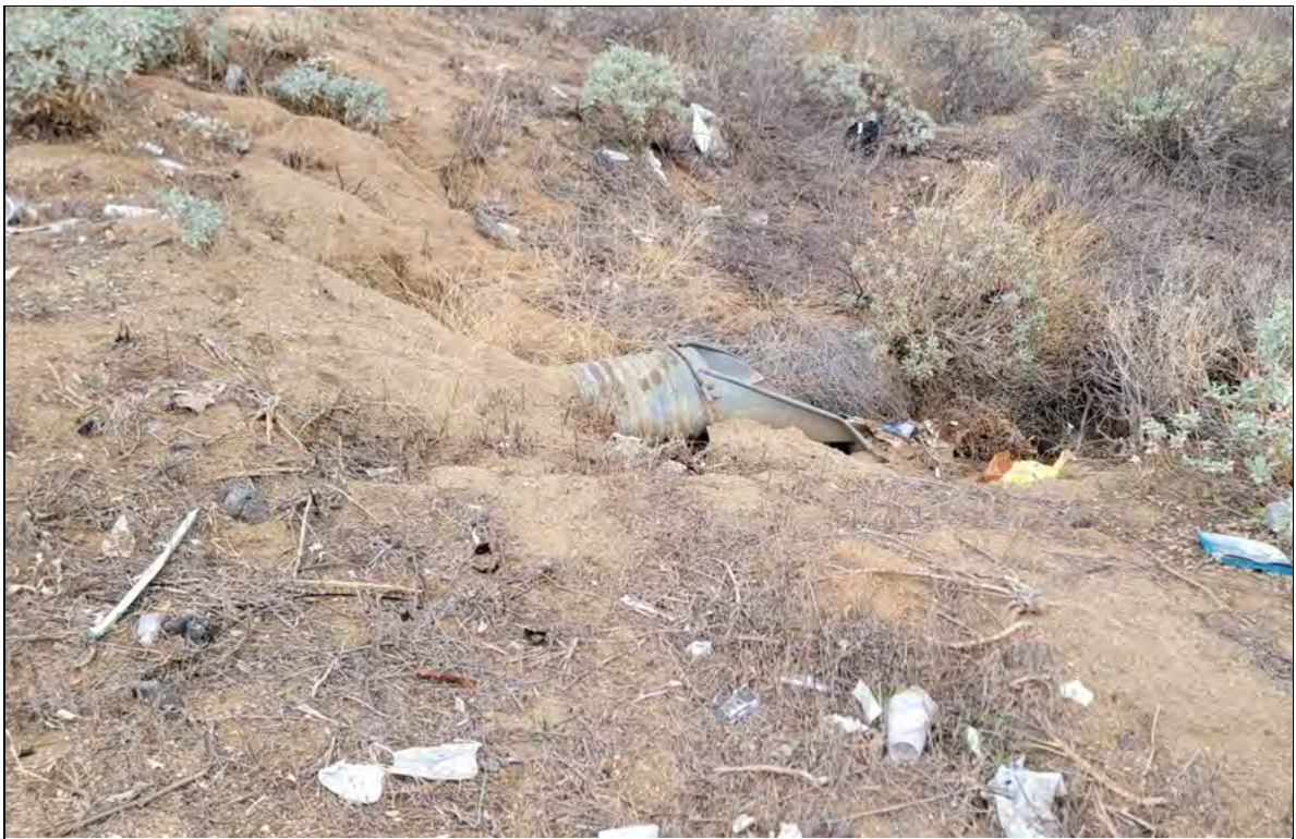
Photograph 16: View of eastern outlet of EF1 culvert, downstream and east of Moreno Beach Drive. Photo depicts existing 30" corrugated metal culvert which will be replaced with an appurtenant facility which will include an energy dissipater which consists of a headwall, rip-rap, and 18-inch storm drain and culvert.
