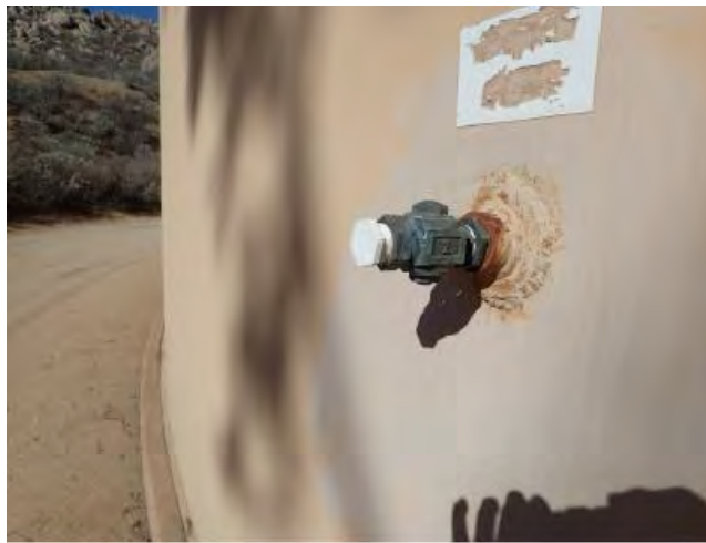
Figure 16: One water tap penetration with minor corrosion around the penetration
