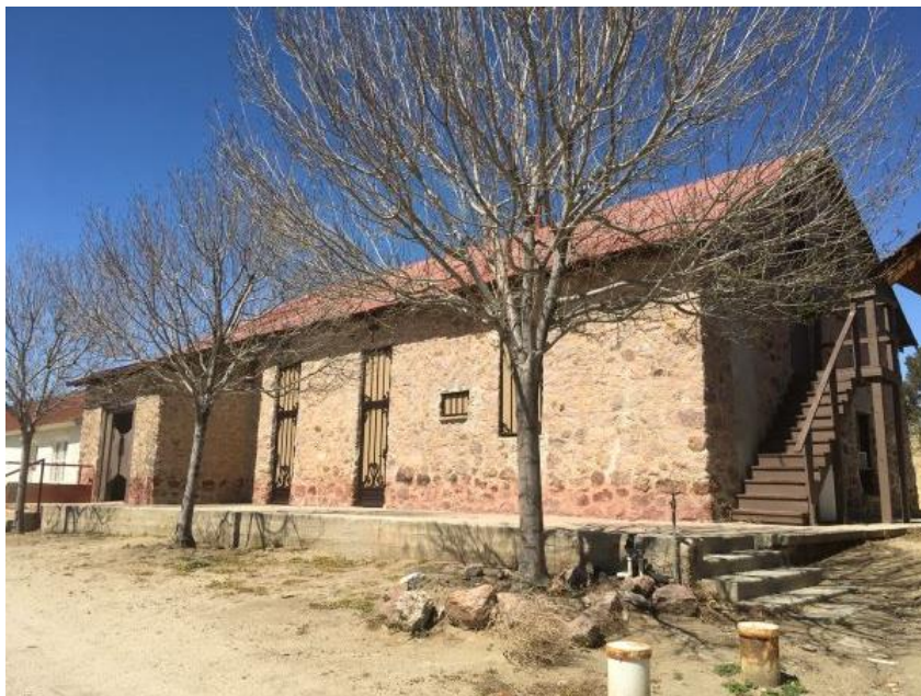
Photograph 3. Primary (south) and east elevations of Building H1 (the town hall), looking northwest
