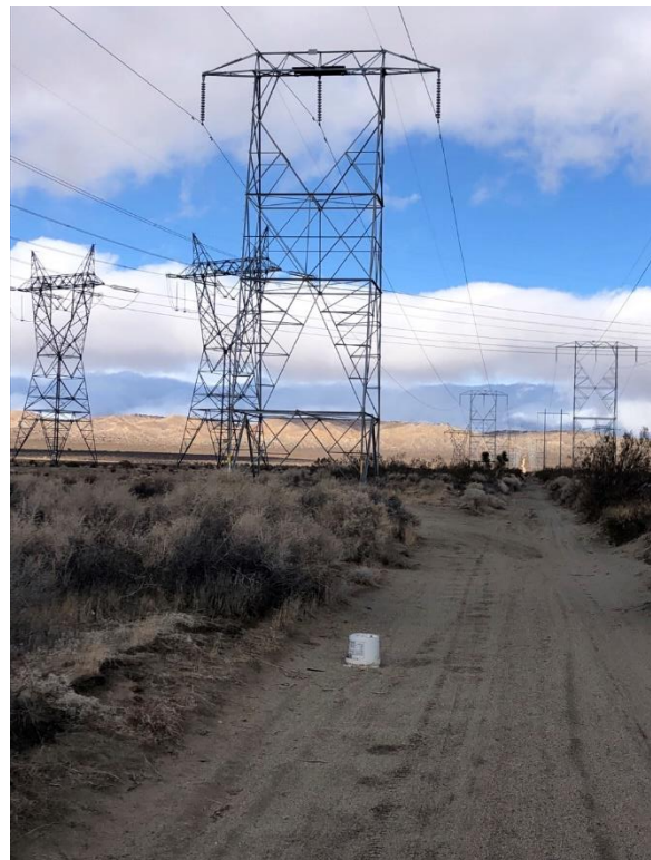
Plate 6-5. View of two SCE Vincent (Big Creek No. 3) 220-kV Transmission Line towers, lefthand side of photograph, facing west
