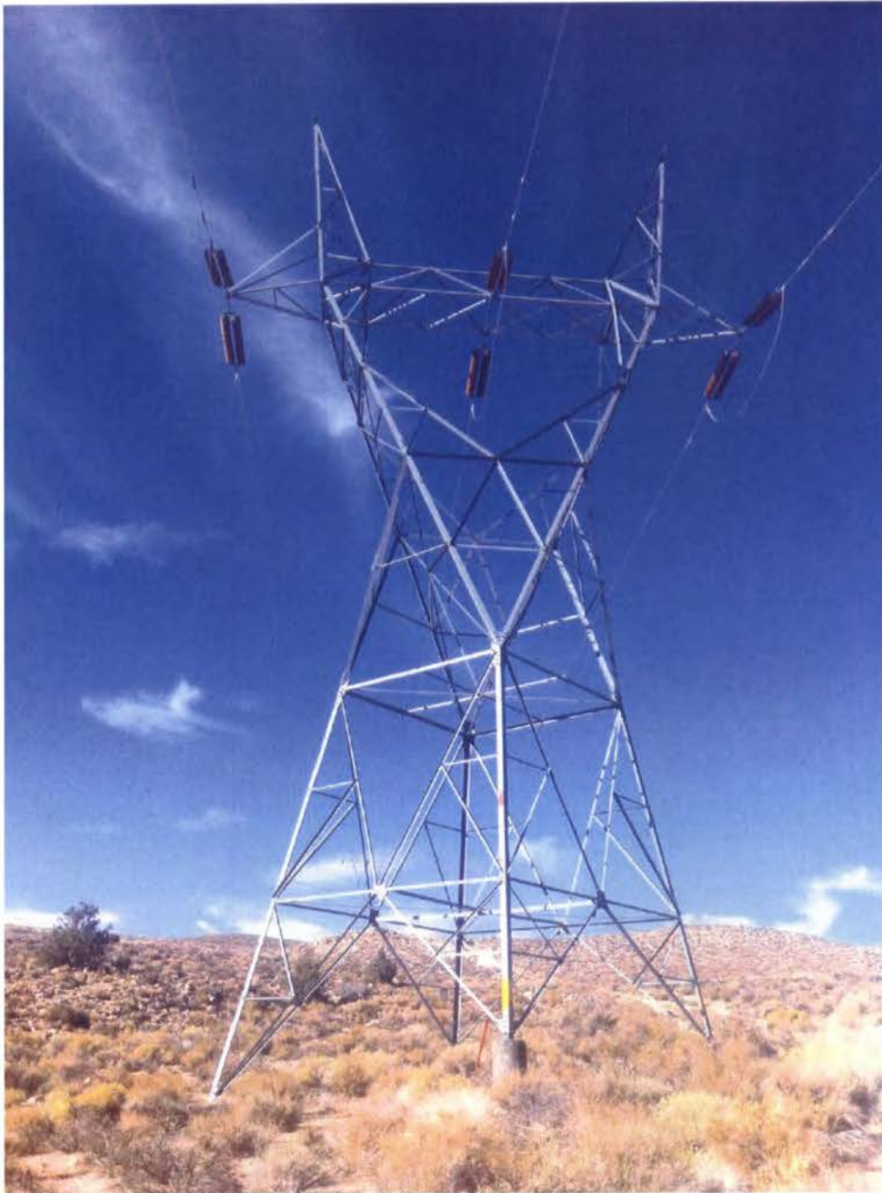
Typical original "dead-end" tower style on the OWE line.
