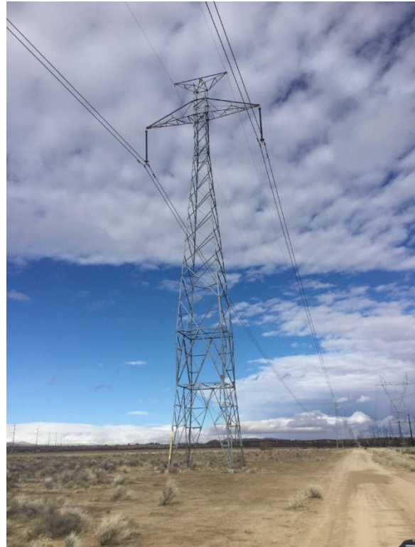
Plate 6-2. Typical Self-Supporting Tower of the LADWP Pacific Intertie 500-kV Transmission Line
