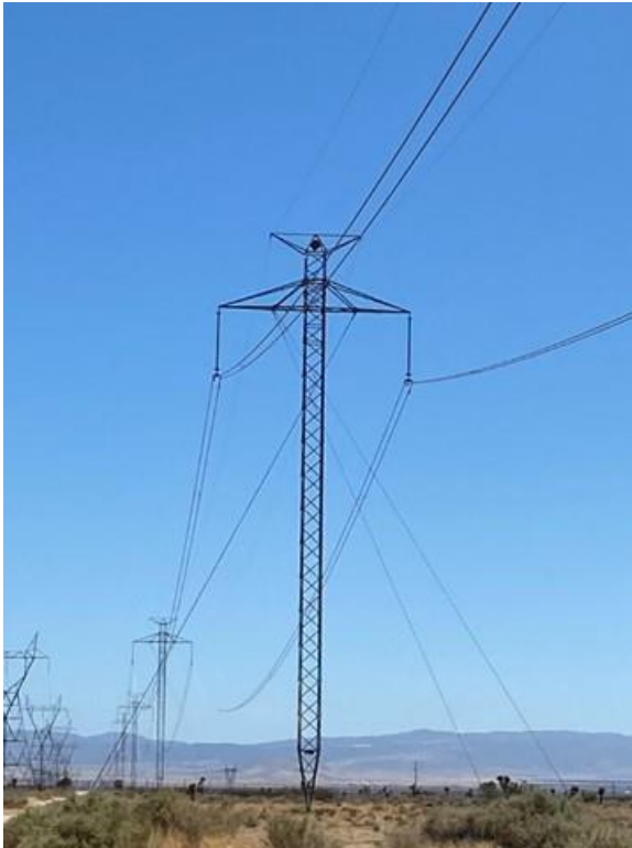
Plate 6-1. Typical Guyed Tower of the LADWP Pacific Intertie 500-kV Transmission Line
