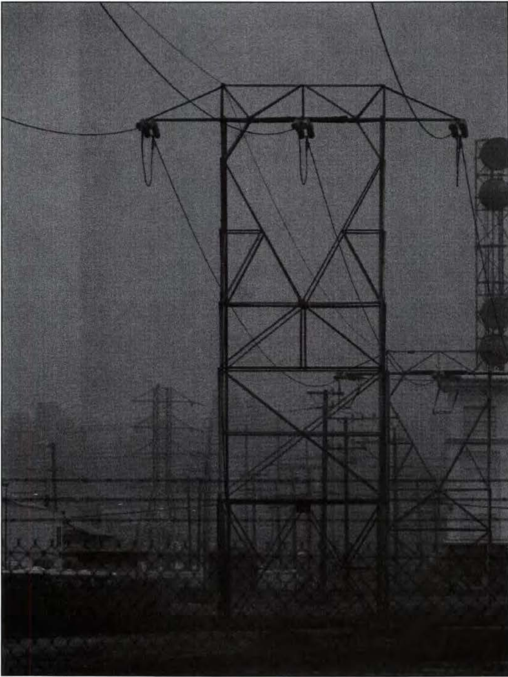
Tower Type #2: Dead End (Anchor) Vincent Tower with Vertical Leg Extension (Mile 147-T1).
