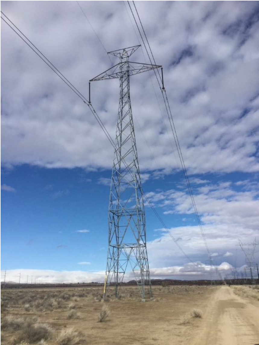
PDCI Transmission Line (left) showing typical self-supporting tower, view north. December 2021.
