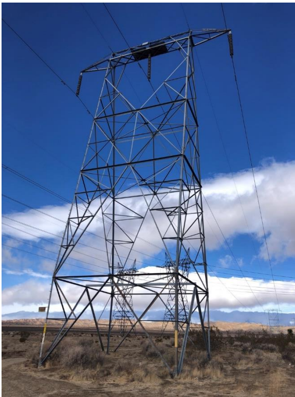
Plate 6-4. Typical tower of SCE Vincent (Big Creek No. 3) 220-kV Transmission Line
