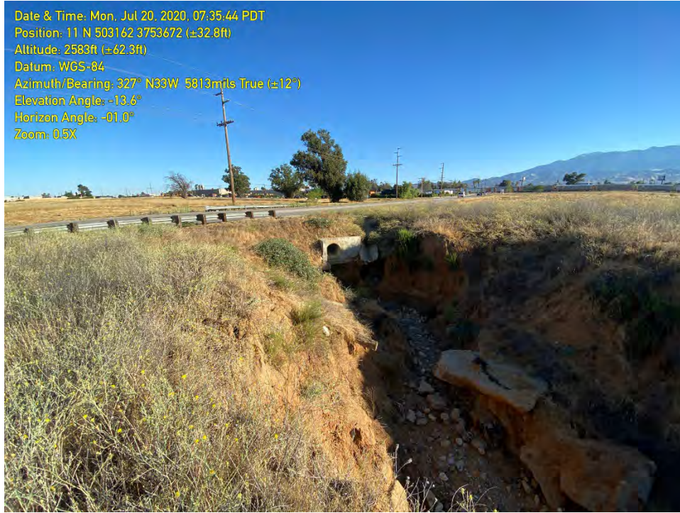
PHOTOGRAPH 1: The upstream portion of Feature A where the culvert begins the feature beneath Pennsylvania Avenue.
