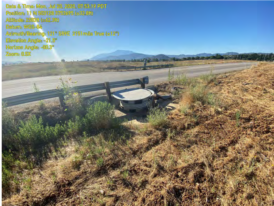
PHOTOGRAPH 3: The westside of Pennsylvania Avenue where storm runoff entered a standpipe connected to the culvert where Feature A began.
