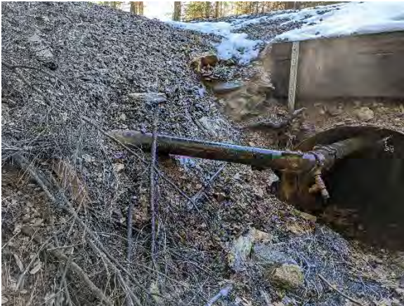
P01 – Broken water pipe in OW08 looking south
