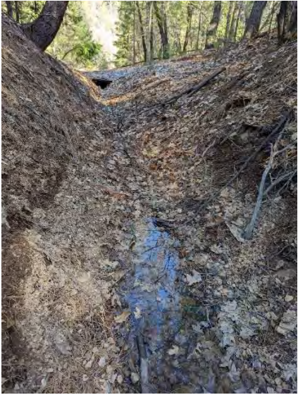
P01 – OW08 looking north (containing standing water from leaking pipe)
