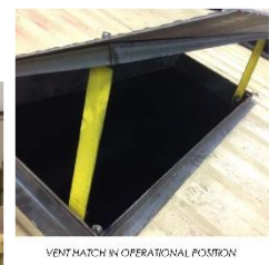
VENT MATCH IN OPERATIONAL POSITION
