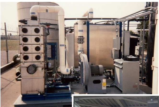
Multi-Phase Extraction System Equipment
