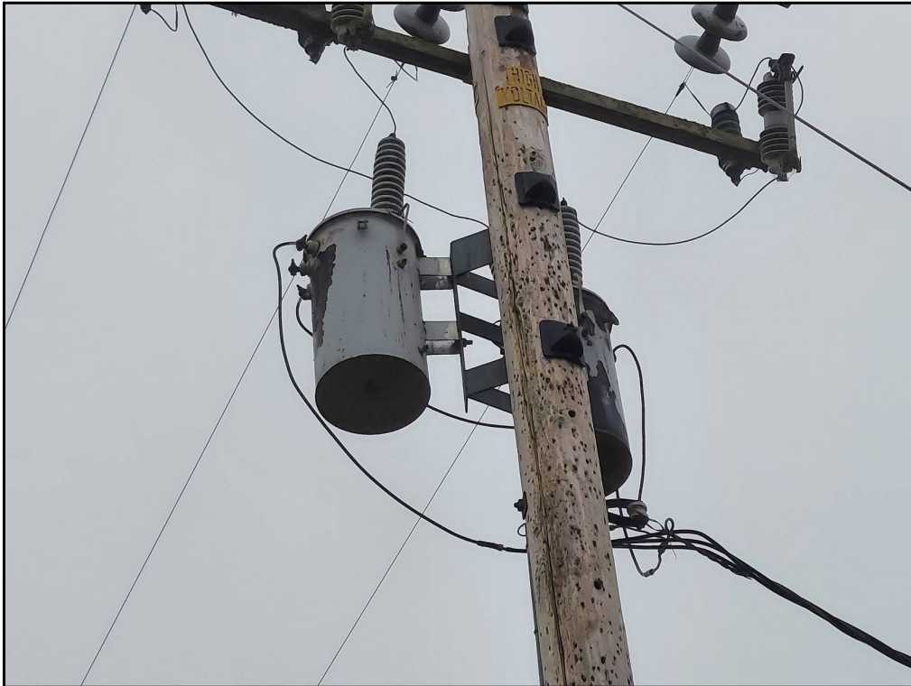
5 : View of the pole-mounted transformer on the site. No signs of leaks or spills were noted.
