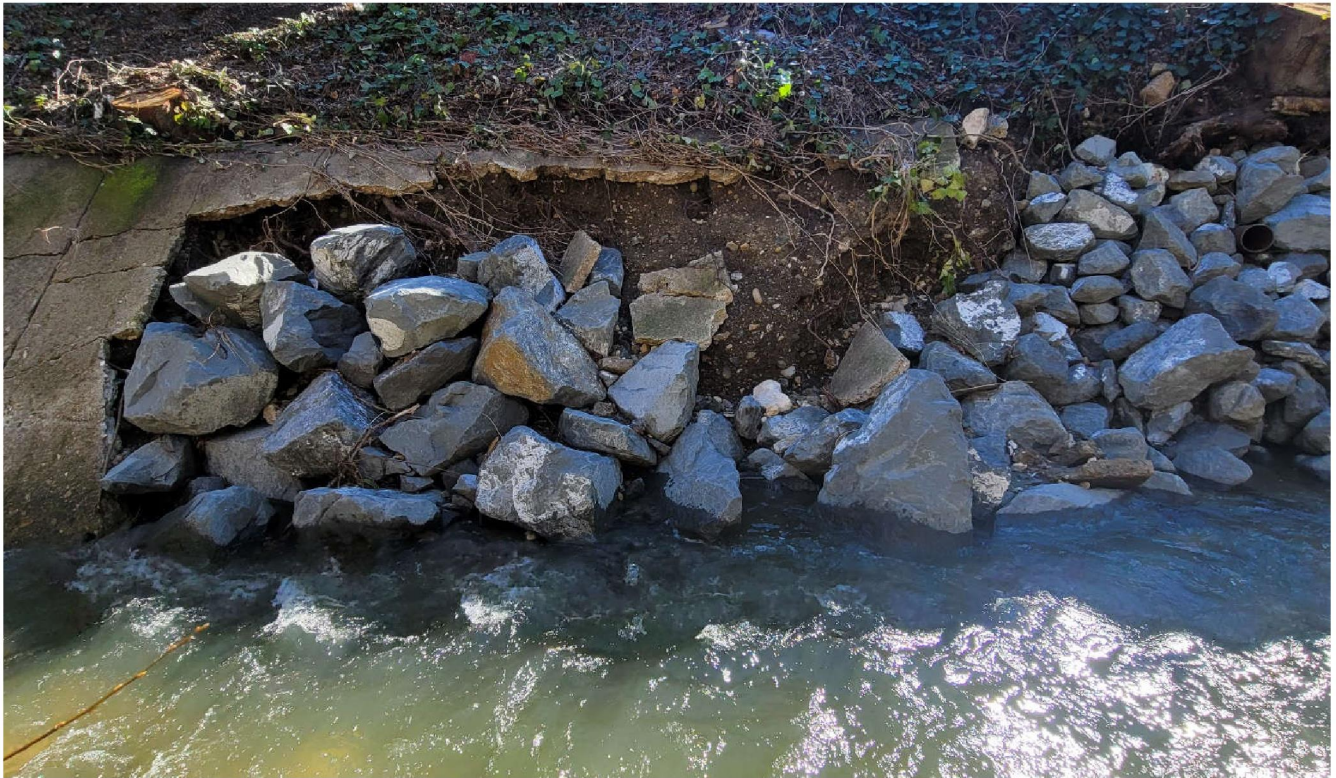
Photograph 3. View of the south bank of San Luis Obispo Creek where the concrete infrastructure has been damaged by rain events in December 2022 and January 2023 (facing south, January 26, 2023).
