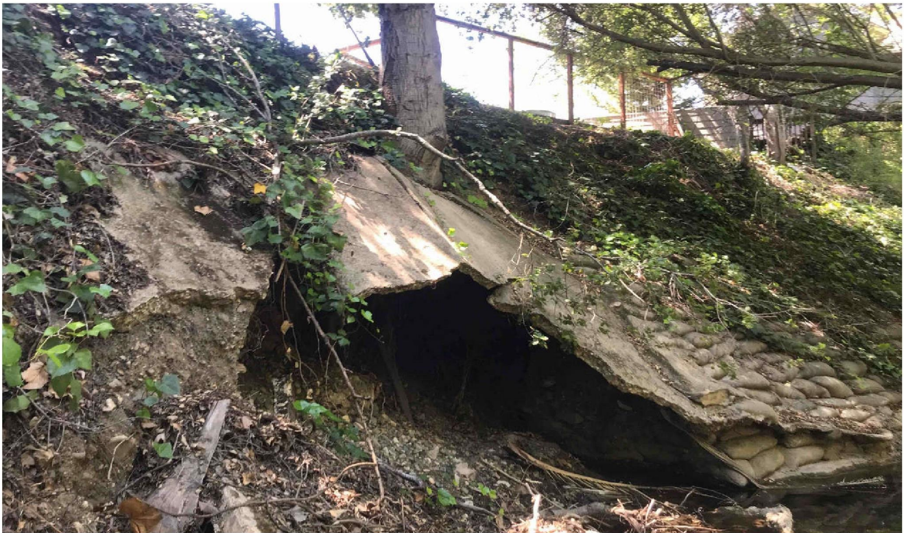
Photograph 1. View of the south bank of San Luis Obispo Creek where the concrete infrastructure has been undercut and eroded by water flow (facing south, May 3, 2022).
