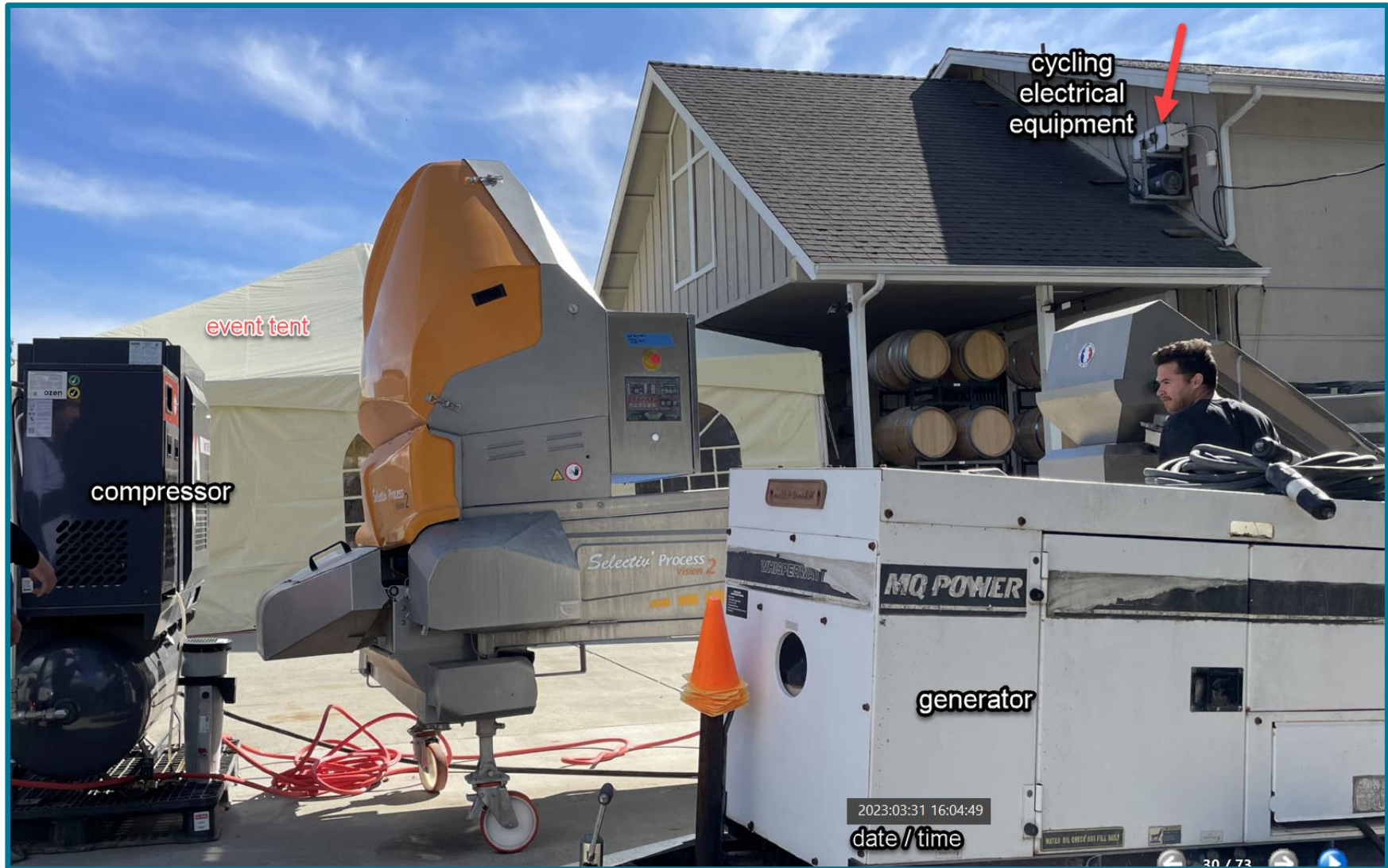
Figure 9: Photo 2 of equipment measured including generator in foreground, tent in background
