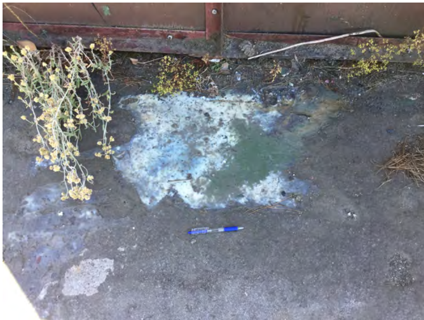
Photograph 10: White staining on asphalt in "Battery Pickup" area with pen for scale.
