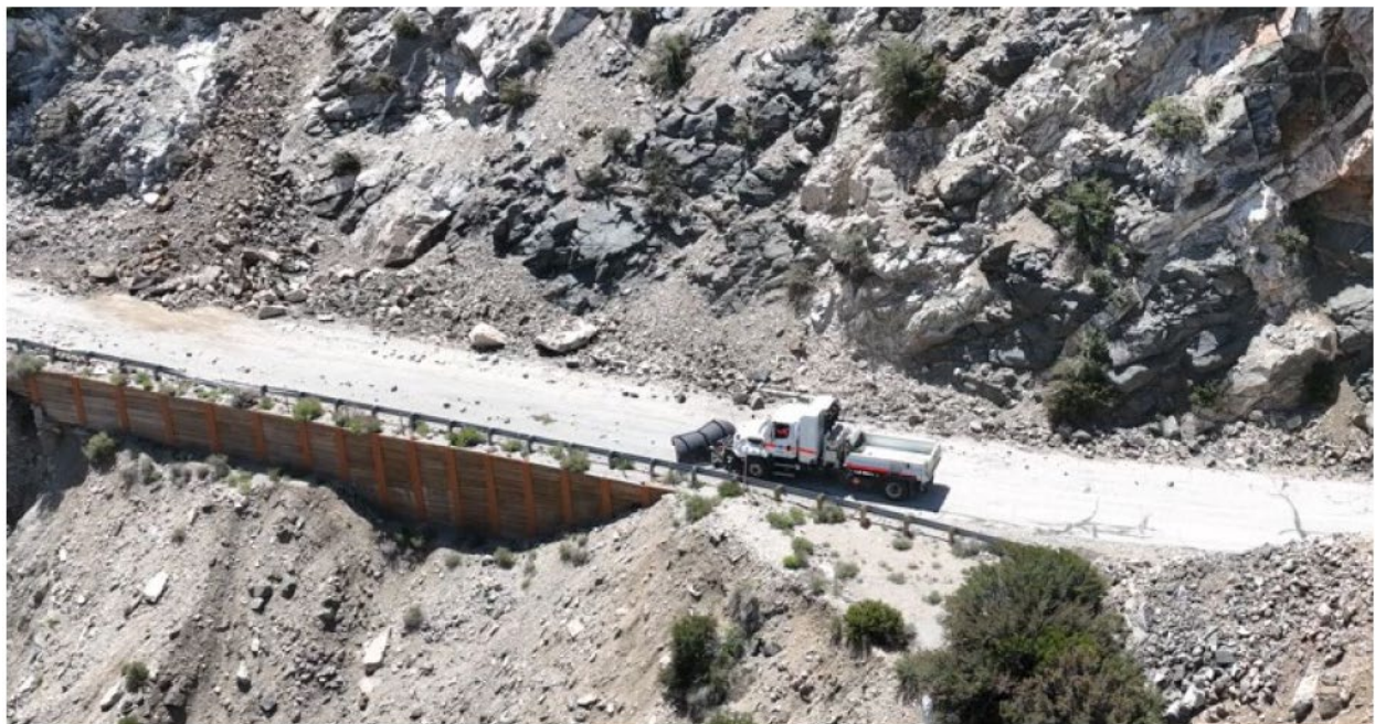
Example from SR-39. Retaining walls should be colored to match existing rock or nearby structure aesthetic treatments.
