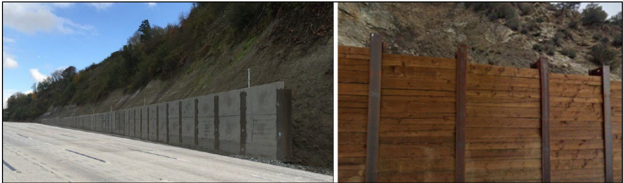
Catchment Wall examples: colored concrete and steel posts (left), and timber lagging and steel posts (right).
