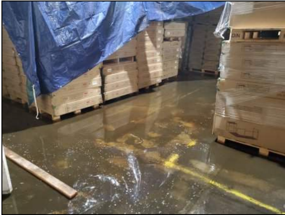
View of standing water due to roof leak in 717 E State St.
