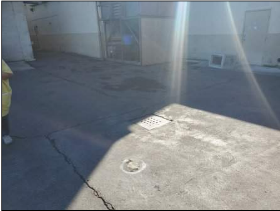
View of typical storm drain grate as observed on north side of warehouse building in western portion of Property.
