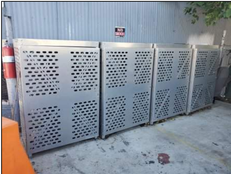
View of propane canister storage on west side exterior of service/storage building.
