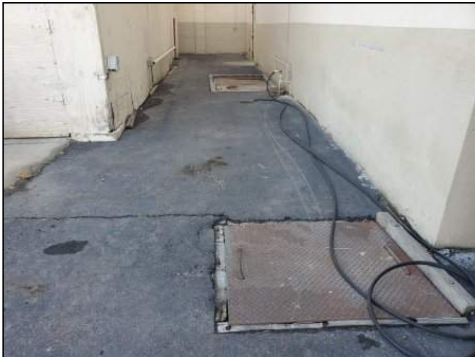
View of vaults located on north side of warehouse building on west side of Property.
