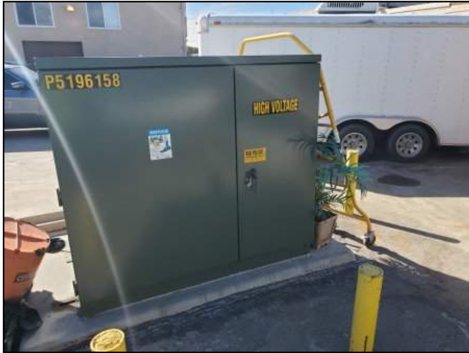
View of pad-mounted transformer at AG Construction yard.
