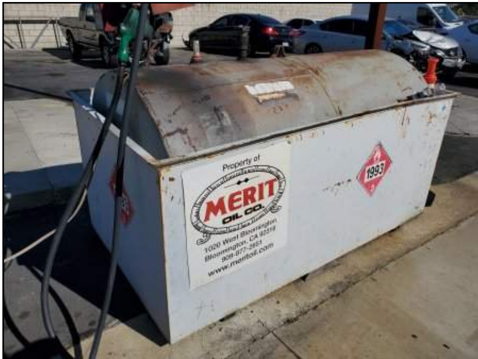
View of 500-gallon diesel AST at 810 E Main Street tow yard.
