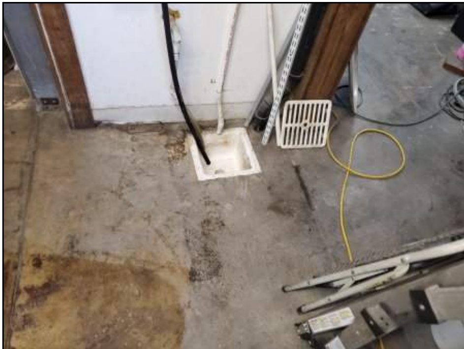
View of floor drain at Strum Brewing.
