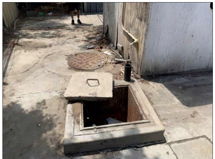
60. Property 7 potential concrete sump adjacent to the former auto repair facility building, view facing south.
