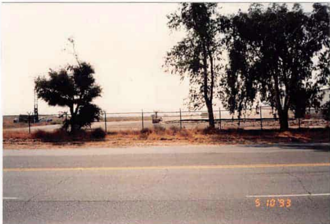
VIEW OF NORTH AIR FORCE BASE FROM SITE SHOWS COVERED EVAPORATION POND COVERED BY TARP AND CDM FEDERAL INSTALLING MONITORING WELL.
