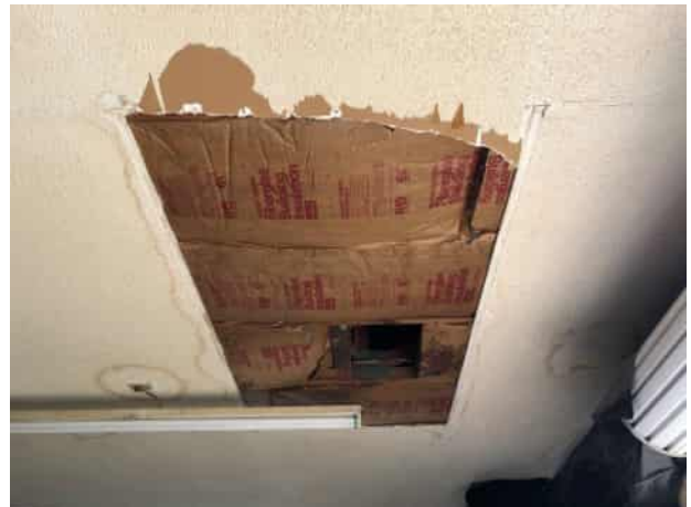
12.View of water damaged drywall cutout from the ceiling.
