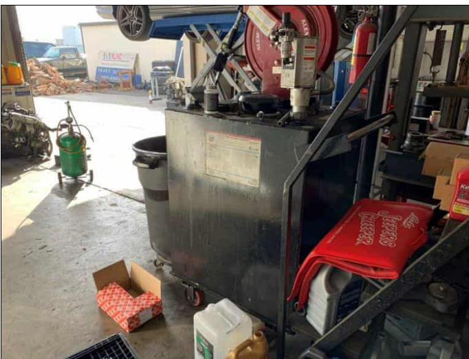
89. 89. Property 11, motor oil AST in central portion of the service building, view facing southeast.
