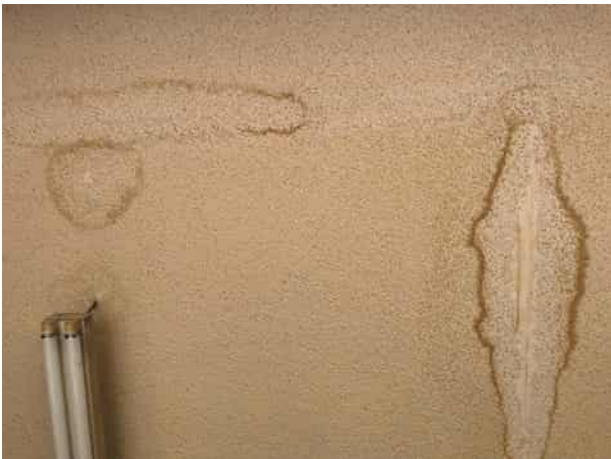
11.View of water damage on the acoustic sprayed ceiling.
