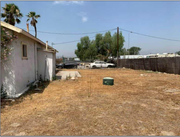
49. Property 7 septic tank on the north side of the residence on the northeast corner of the property, view facing west.
