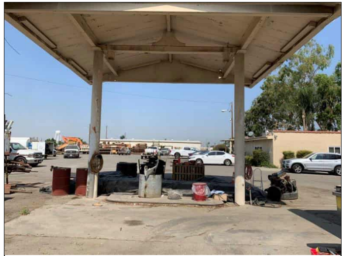
10. Property 2 former UST area on the northeastern portion of the property, view facing west.
