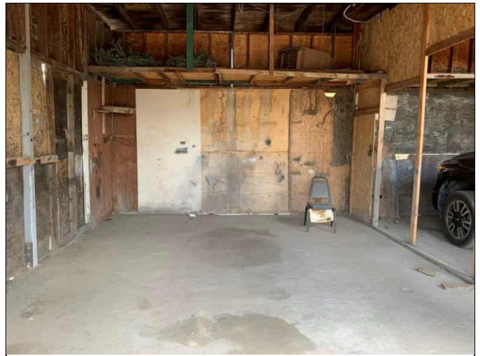
52. Property 7 (central portion of the subject property) structure interior, view facing north.
