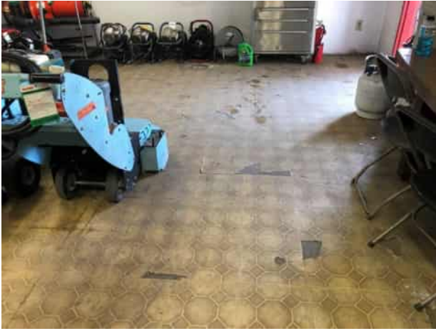
13. View of damaged and chipped floor tiles in the southern building.
