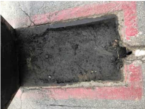
11.View of the stormwater drain collection area full of mud.
