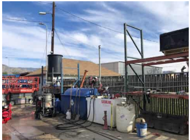
6.View of the diesel and gasoline ASTs on the south parcel.
