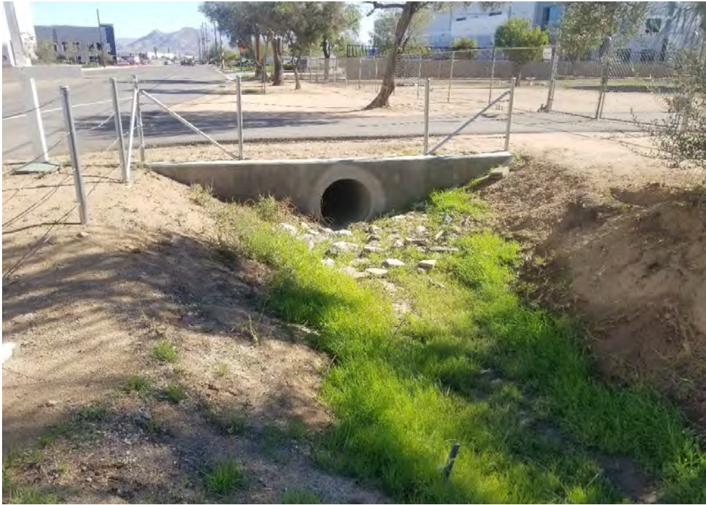
Photograph 6: View depicting eastern terminus of roadside ditch, immediately south of Rider Street.
