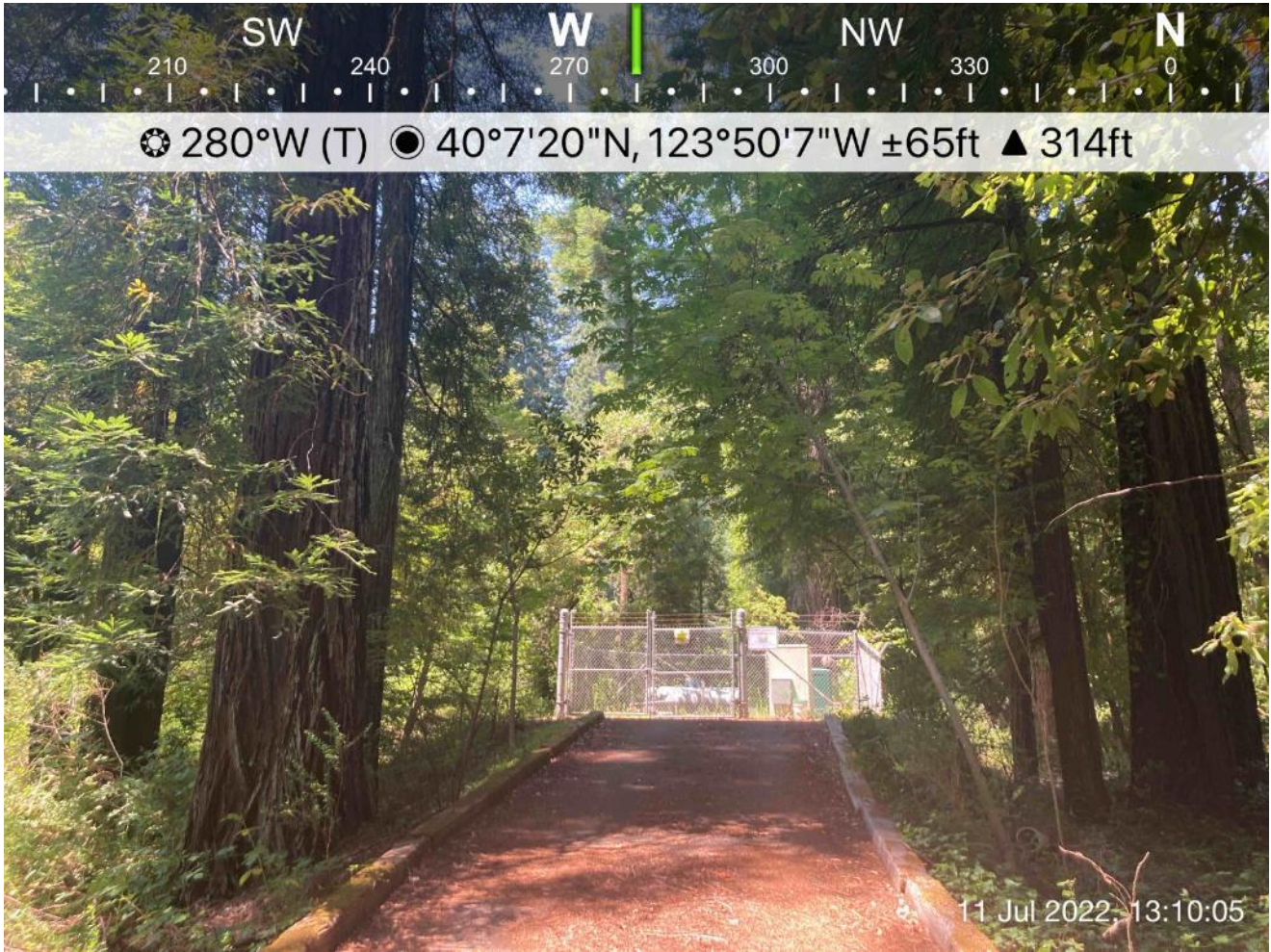
Image B8. Example of one of the pump stations in a residential area, with established coniferous trees and understory.
