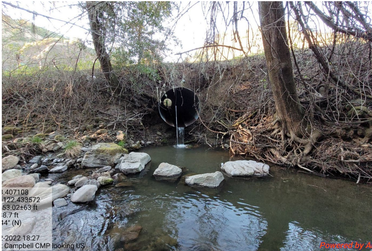
Photo 1. Outlet of the Dry Creek Road Culvert conveying flows from Campbell Creek to Dry Creek.
