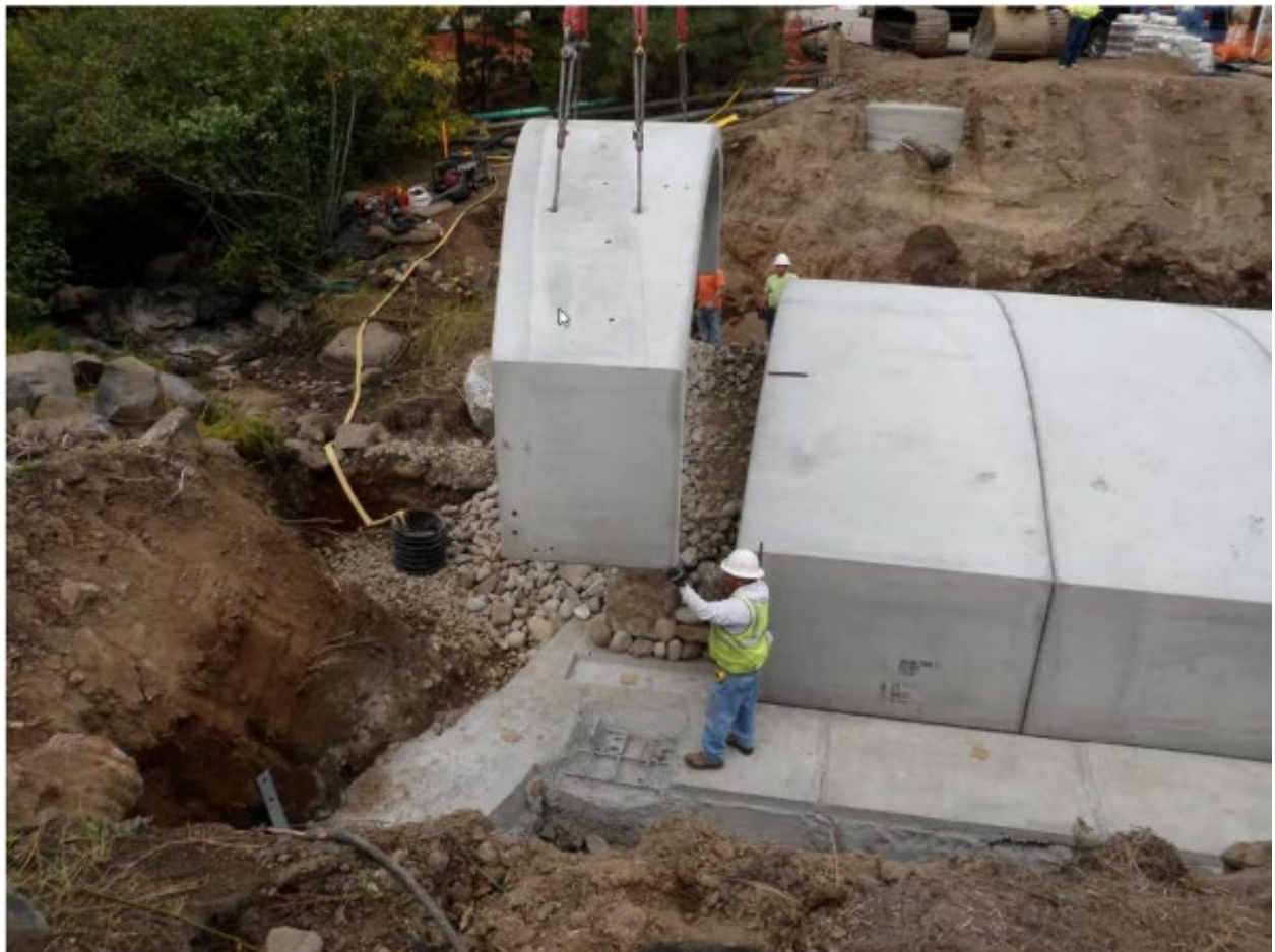
Photo 3 Installation of a Bottomless Arch Bridge Precast Culvert along Third Creek in Incline Village, Nevada
