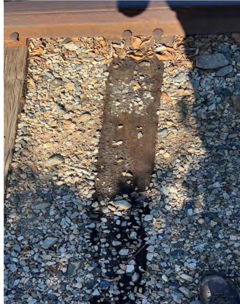
Photograph 2. Railroad tie along the water treatment chemical delivery railroad tracks discolored with a creosote-like material.
