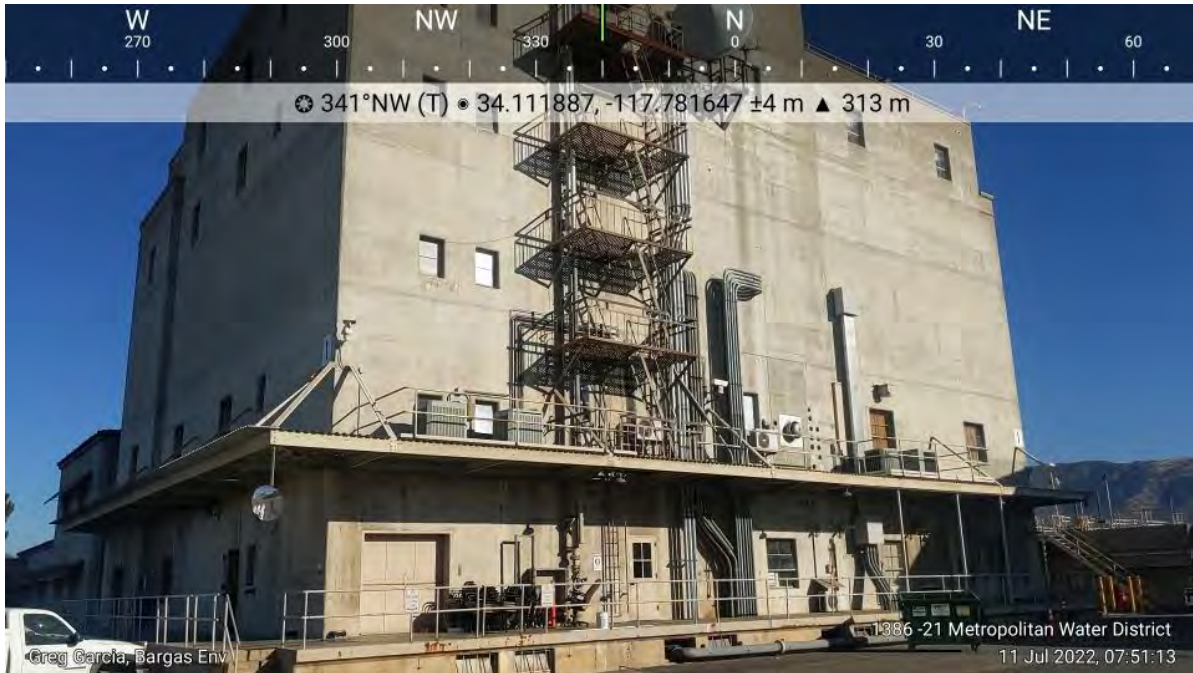
Photo 3. Representative photo of the Administration and Control Building (east-facing building) proposed to undergo various building improvements. Photo looking northwest from inside the Plant.
