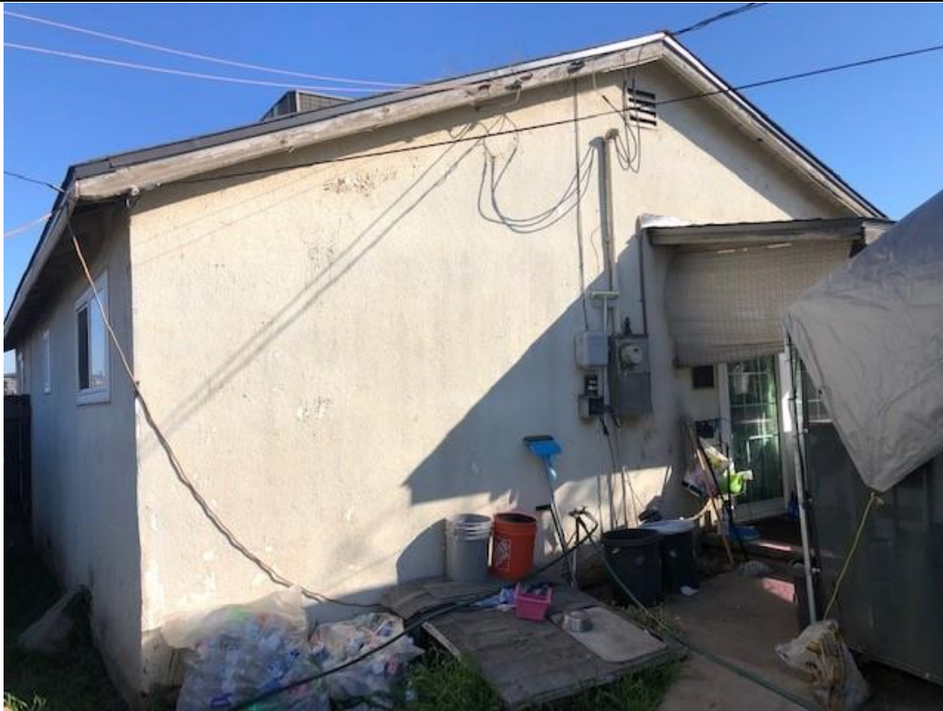
C) View looking north, northwest of the west (left) and south facing facades of the residence. 2/28/22. Acc. #2022IMG5823
