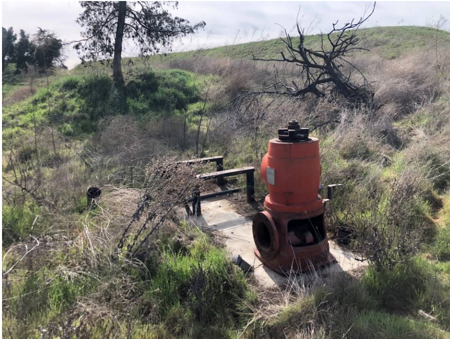
View of a possible pump on the Diocese of San Bernardino Property likely associated with a water well, observed at the edge of the area where structures were formerly present.
