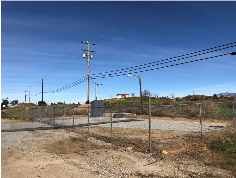
View of the Yucaipa Valley Water District lift station located adjacent to the Subject Properties along Calimesa Boulevard. Pole-mounted transformers were observed along the southwest edge of the Subject Properties.
