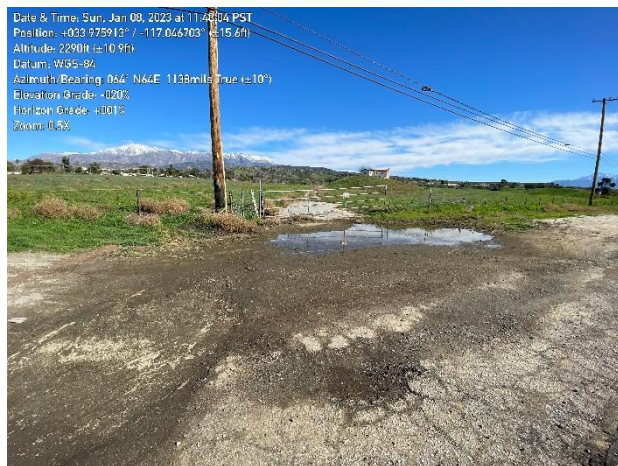
Ponding water in offsite area along Calimesa Boulevard, northwestern portion of site facing east-northeast (01.08.2023).
