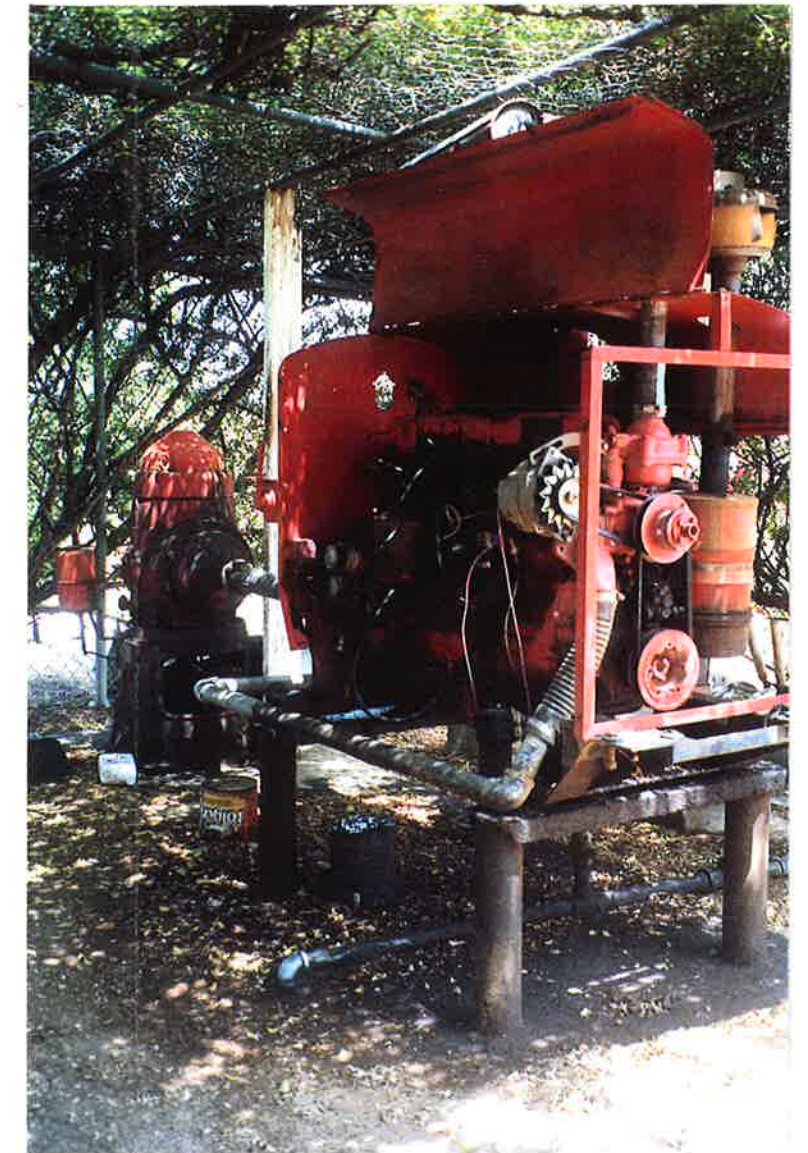
Pump with associated motor for active well located on-site.
