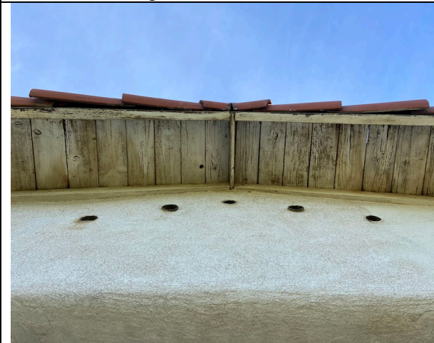
Closer view of the Spanish tile roof of the abandoned residence, and the crevices that contain suitable roosting habitat for bats.
