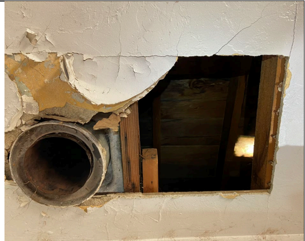
View of the attic access point in the ceiling on the inside of the abandoned residence. Access points are also available for bats along the exterior of the house.
