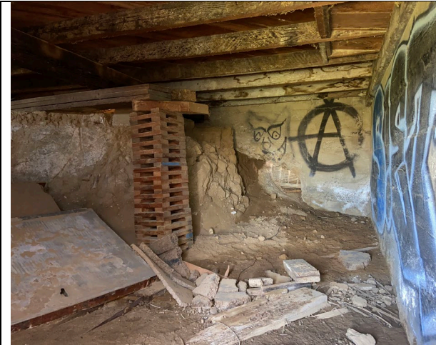
View of the basement beneath the abandoned residence. Some scattered guano was observed along the walls of the basement, indicating some use by bats for roosting.
