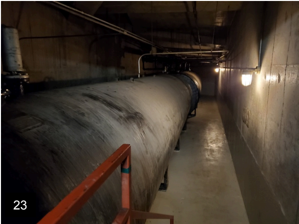
23 8,800-gallon diesel ASTs
