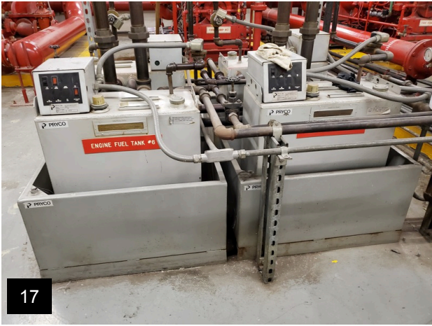
17 Day tanks for fire pumps
