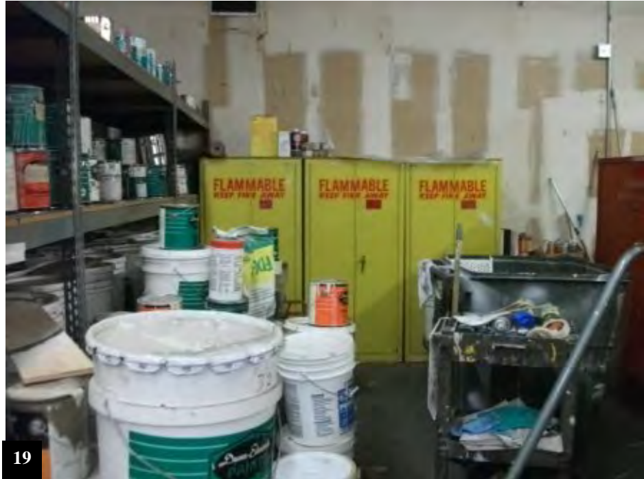
Chemical storage cabinets in paint shop
