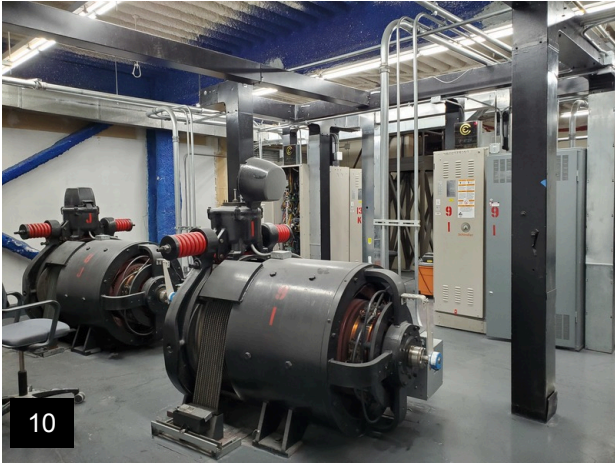
10 Traction elevator equipment on roof of office tower
