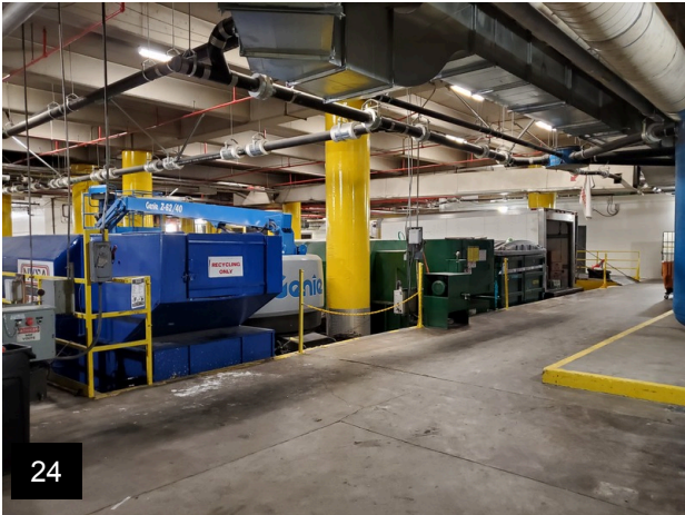
24 Trash compactors at loading dock
