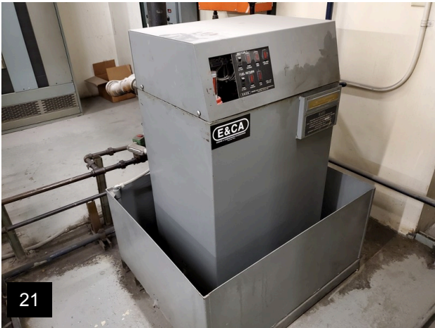
21 Day tank for emergency generator
