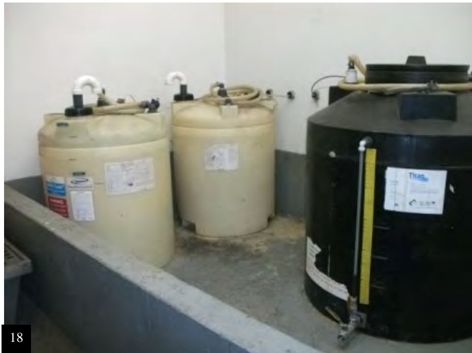
Cooling tower chemicals
