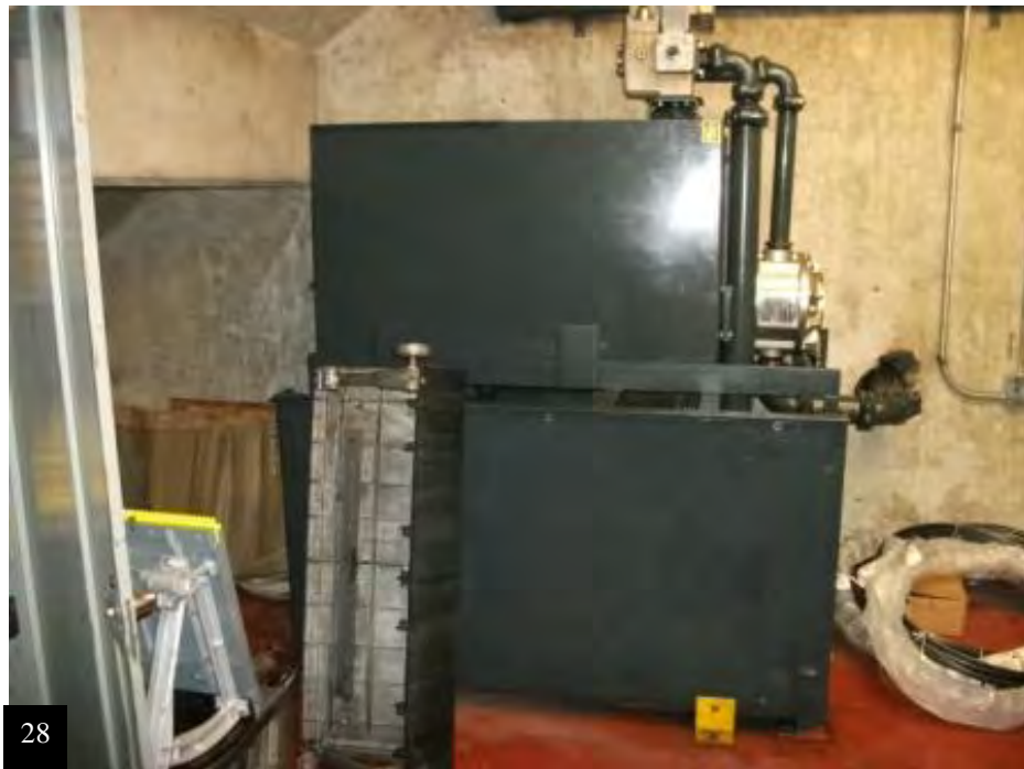
Hydraulic elevator equipment
