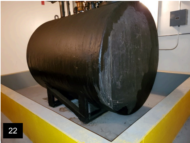
22 1,000-gallon diesel transfer AST
