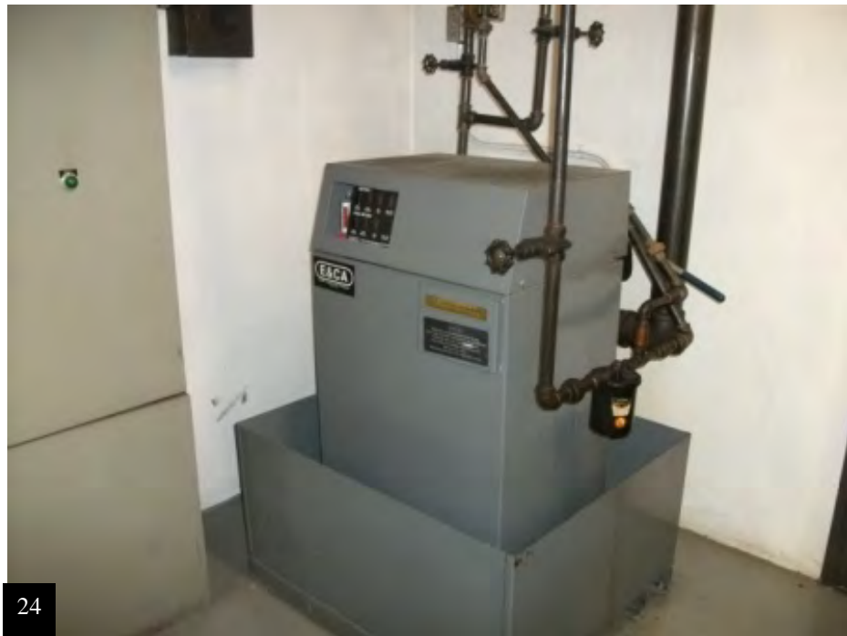
Generator day tank
