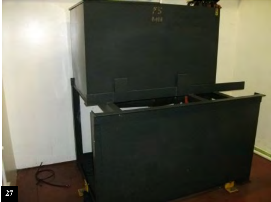
Hydraulic elevator equipment
