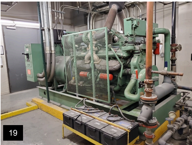
19 Emergency generator for Sheraton Hotel
