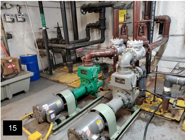
15 Stormwater and sewer sump pumps
