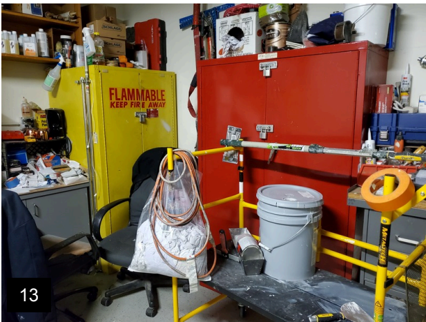
13 Chemical storage cabinets in maintenance area
