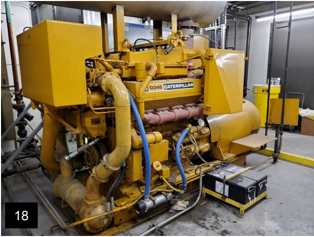
18 Emergency generator for office tower
