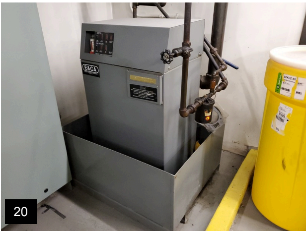
20 Day tank for emergency generator
