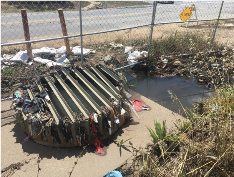
Photo 4: Storm Drain Overflow System (E)
