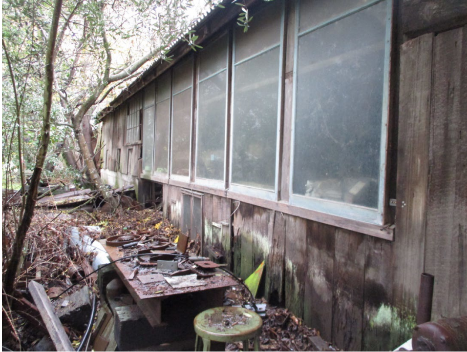
Figure 10. East side of the north elevation of the ca. 1923 walnut barn, with work benches.
