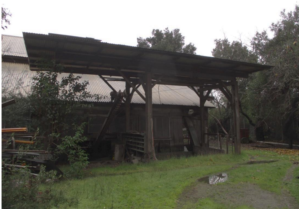
Figure 56. West side of the north elevation of the ca. 1923 walnut barn, showing awning over the pit.
