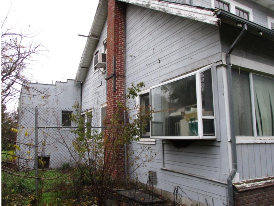
Figure 42. Showing the garden window box and chimney along the west elevation and the second addition, facing northeast.
