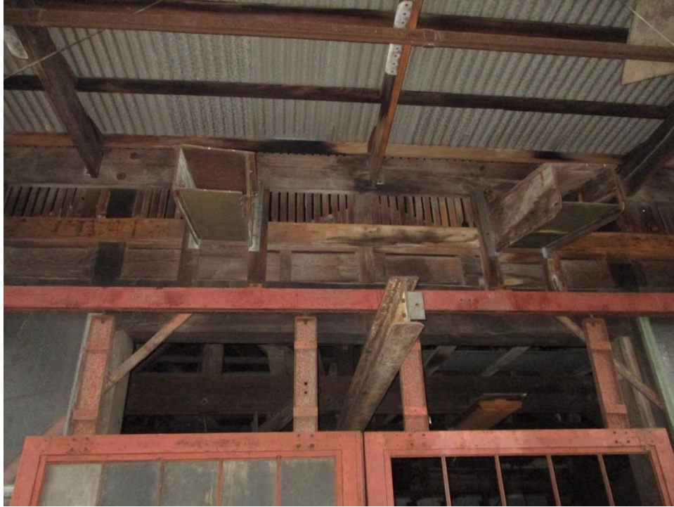
Figure 53. Walnut chutes leading out of garage over main entry on the west elevation.
