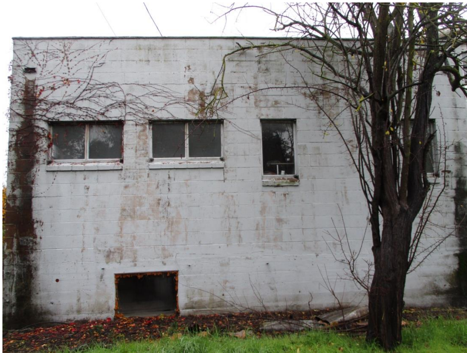
Figure 43. Showing the aluminum windows set within the concrete block wall along the west elevation, facing east.
