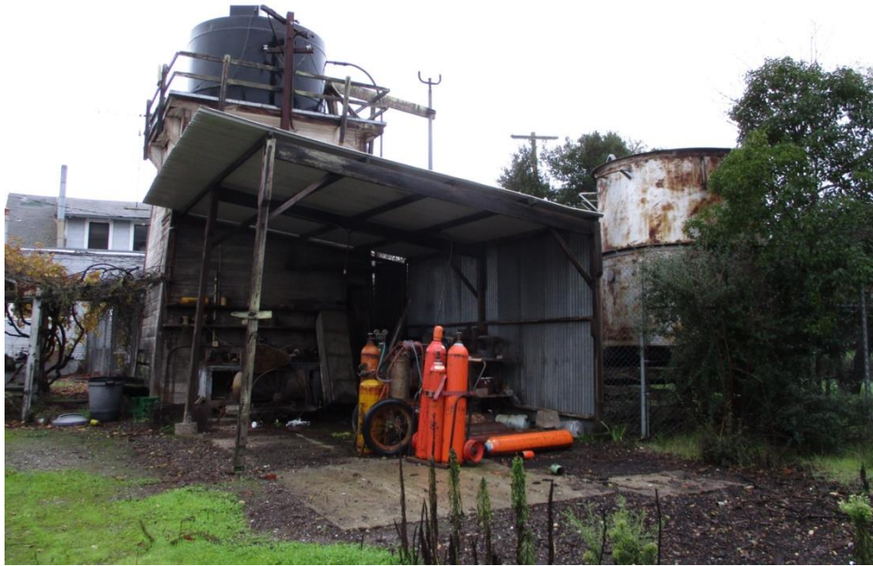
Figure 45. Photograph showing the attached wood structure of tank house 1 (center) and tank house 2 (right).
