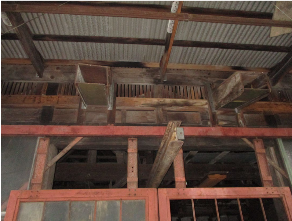
Figure 2. Walnut chutes leading out of garage over main entry on the west elevation.
