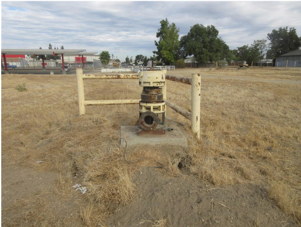
Photo 10: View of the non-operational water well located in the central-western portion of the subject site.
