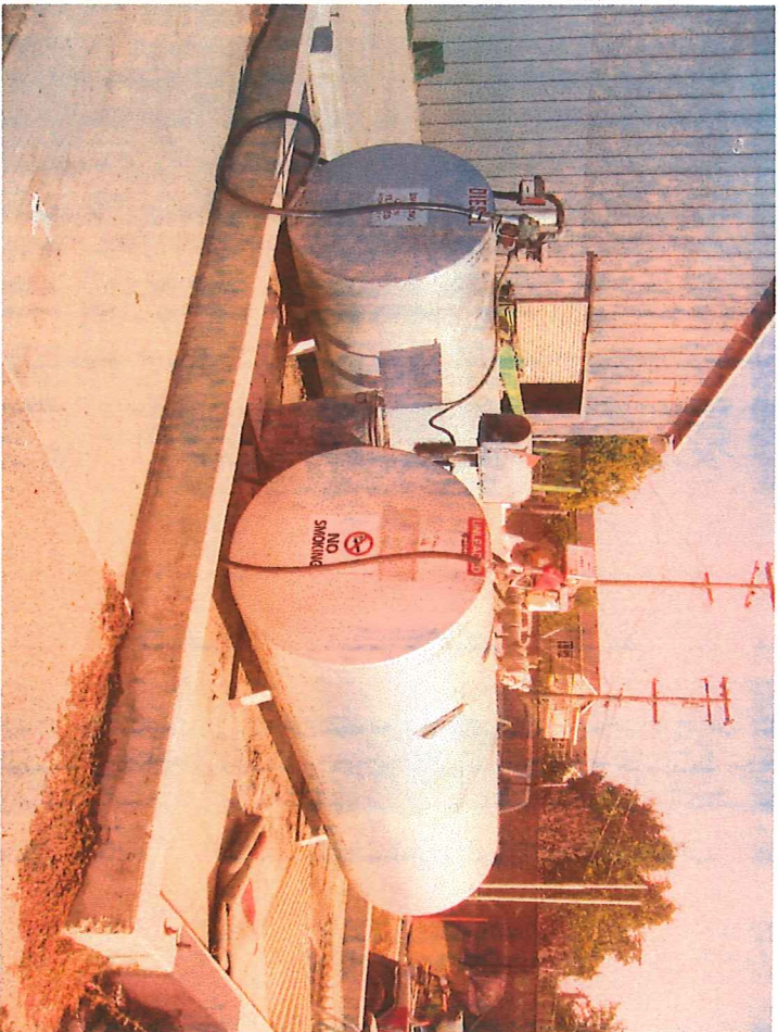
2,000 gallon Regular and Diesel aboveground storage tanks
