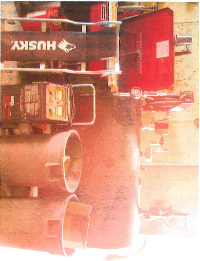
250 gallon motor oil tank and cleaning solvent tank.
