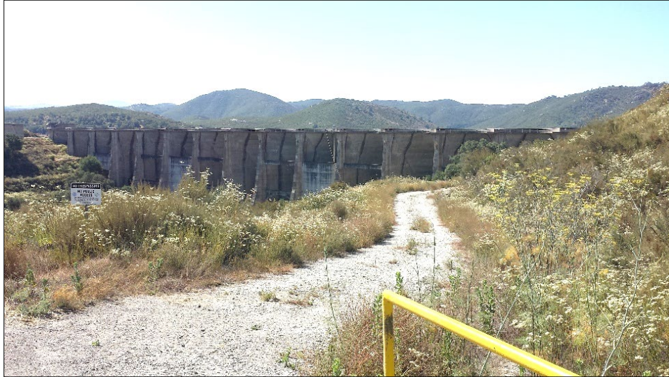
Plate 13. Overview of dam and access road off Sutherland Dam Road. View to the south.
