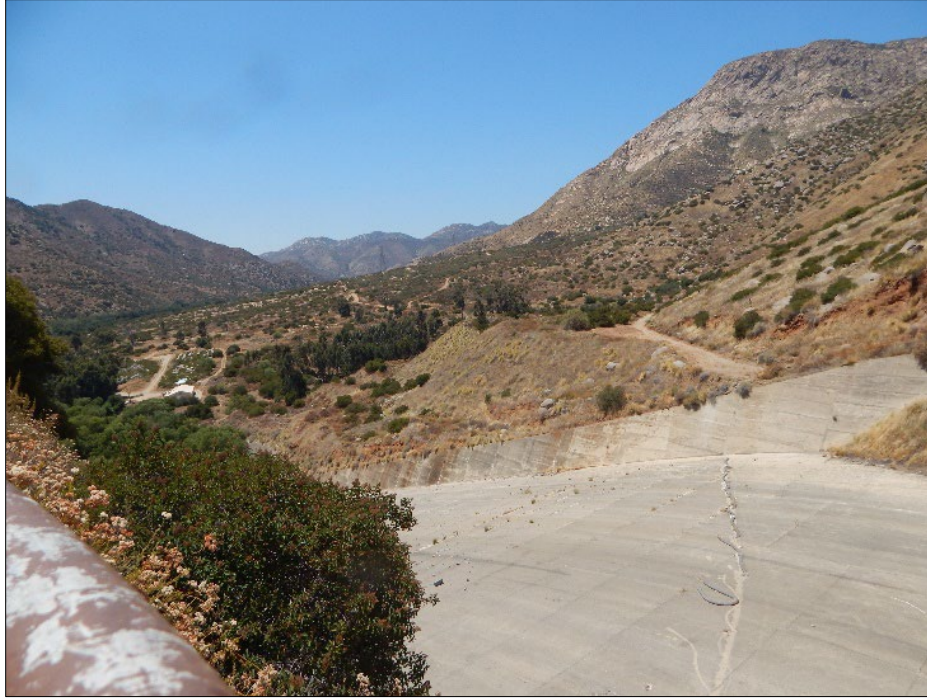
Plate 5. Overview of El Capitan Dam spillway, west side. View to the west.
