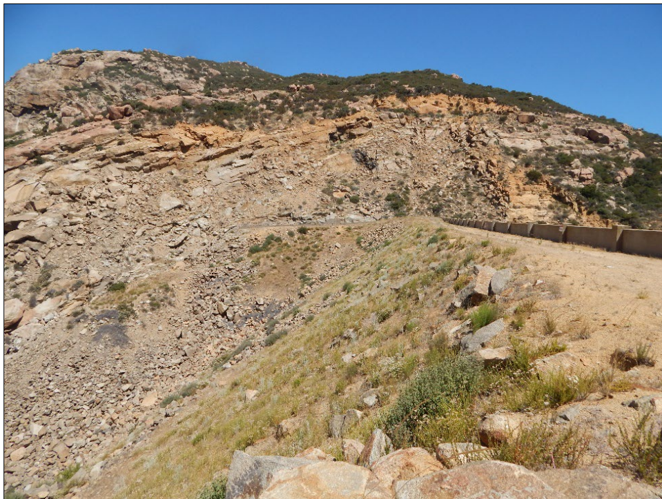
Plate 8. Overview of the Morena Dam spillway and north end of the dam. View to the north.
