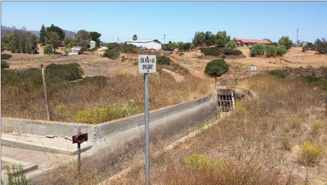
Plate 2. Overview of concrete Conduit section and tunnel entrance. View to the northeast.
